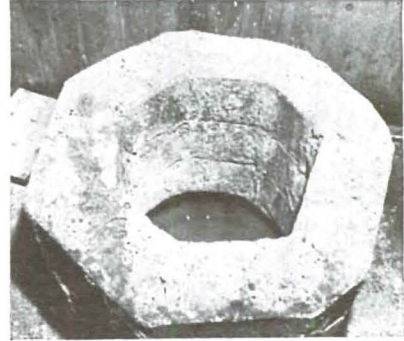
The sump pump well is no longer used. Pump was disconnected months ago. Water still rises to the floor level as can be seen in the above photograph — proving that the floor and walls of the pit are still surrounded by water held back by Aquella.
