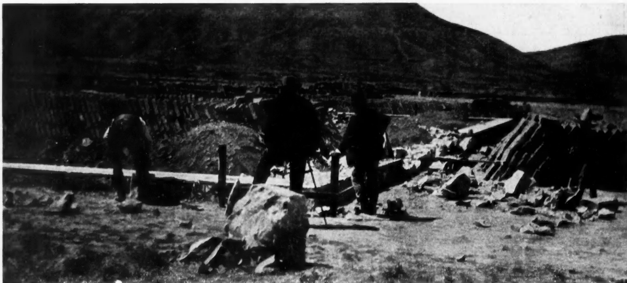
Stone Foundation for Large House with Piles of Adobes Ready to go into the Walls
