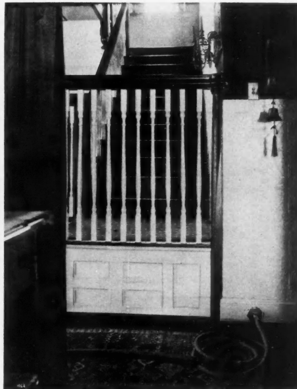
Baseboard Outlet with Air Hose on First Floor of Residence; Equipped With Built-in Vacuum Cleaning System
