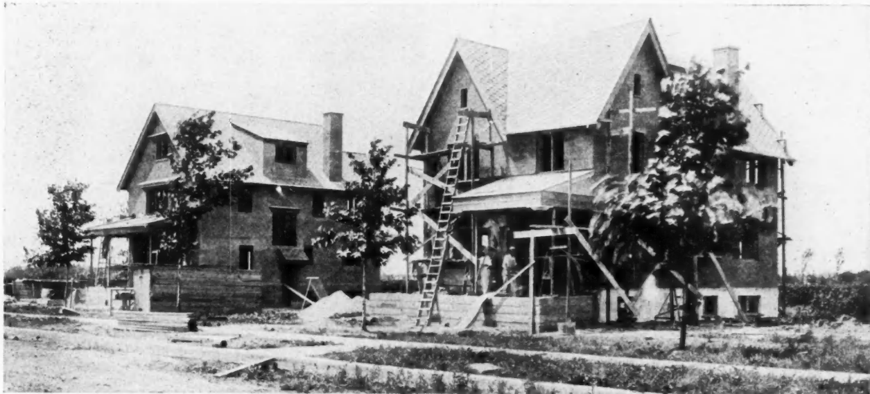
Hollow-Wall Concrete Houses at Bellaire Park, Long Island, New York City Unfinished Porch Foundations Show the Hollow-Wall Feature
