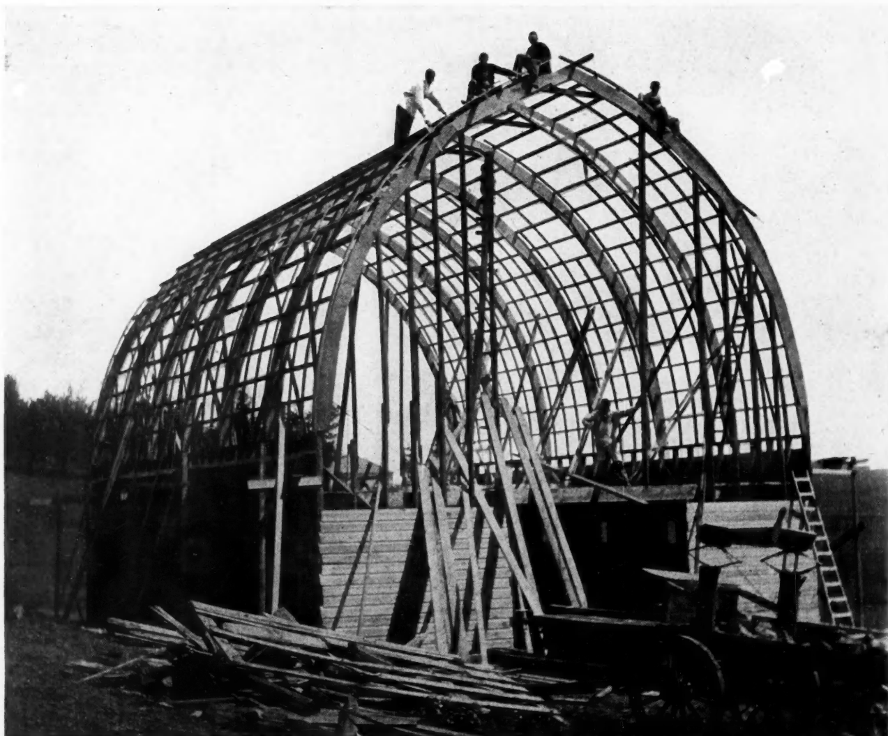
WM. STEINER AND MEN FRAMING GOTHIC ROOF BARN AT JOHNSON, WASH. Curved Rafters are Sawed Out 1 by 12's and Nailed four together.
