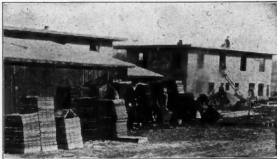
Morrill Steel Forms Used on the "Concrete City" at Nanticoke, Pa., for the D. L. & W. R. R. Co.
