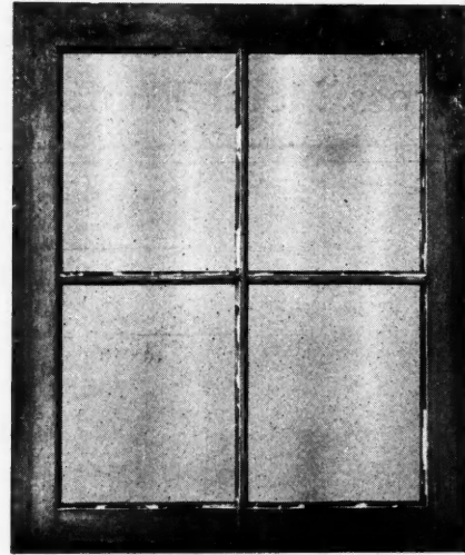
Putty Peels away in a Year or so—A Dilapidated Sight
