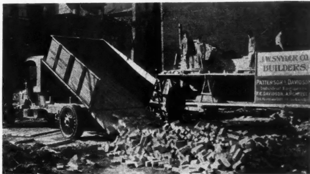
Showing a Pierce Arrow 5-Ton Truck in Use By a Prominent Building Company
