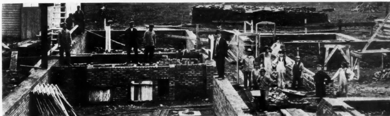
Work Begins on New Fire-Proof Public School Building, at West Mentor, Ohio. The Mettler-Gloyd Co., Contractors.
