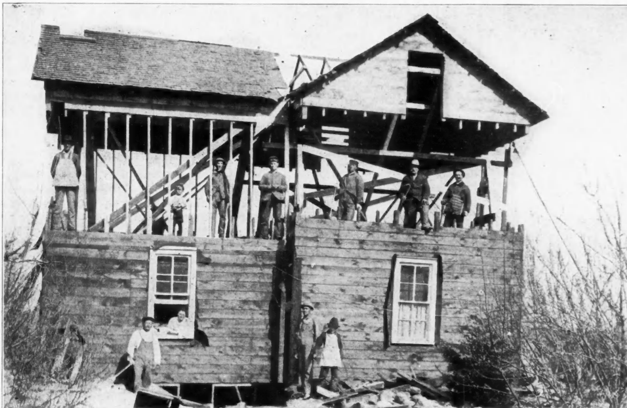
Builder J. T. Reed and his gang at work raising the roof near Armour, N. Dak.
