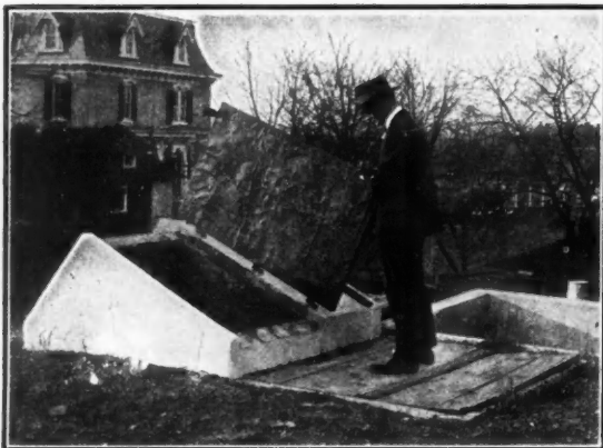
Well Built Little Concrete Pit or Vault for Acetylene Generator.
