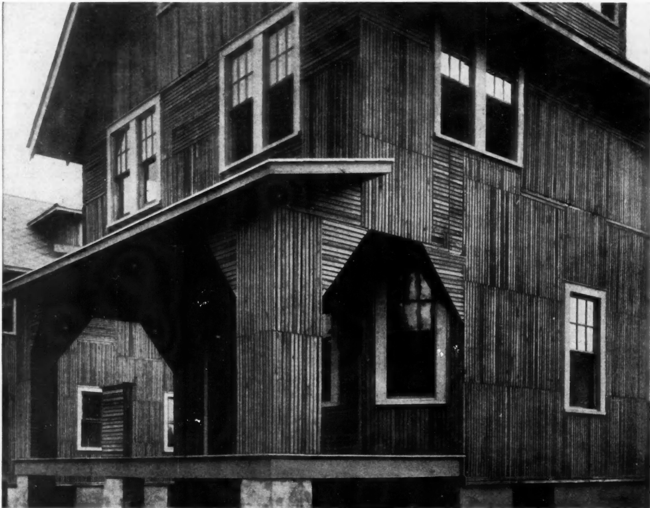
How "Bishopric" Stucco Board Looks on the Wall—All Ready for Cement Plastering. Photo of a Group of Fine Residences Being Put Up by the Passaic Building Co.
