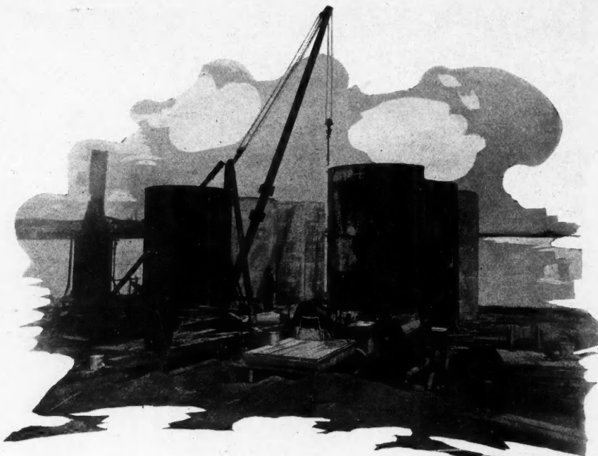
Pouring Intake Pipe Sections at Westport, Baltimore, with Help of two "Wonder" Mixers.
