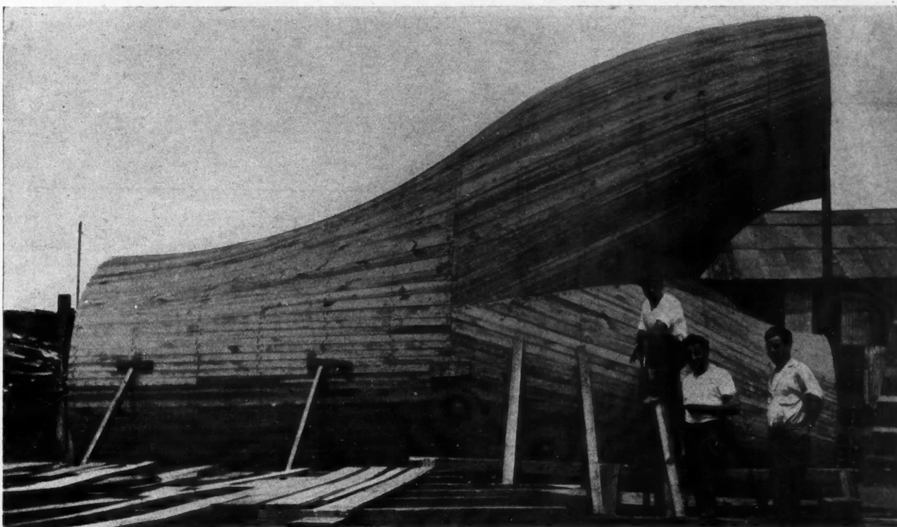
Wood Form of Y Connection in Huge Concrete Sewer at Newark, N. J. Form Designed and Built by F. W. Klauser.
