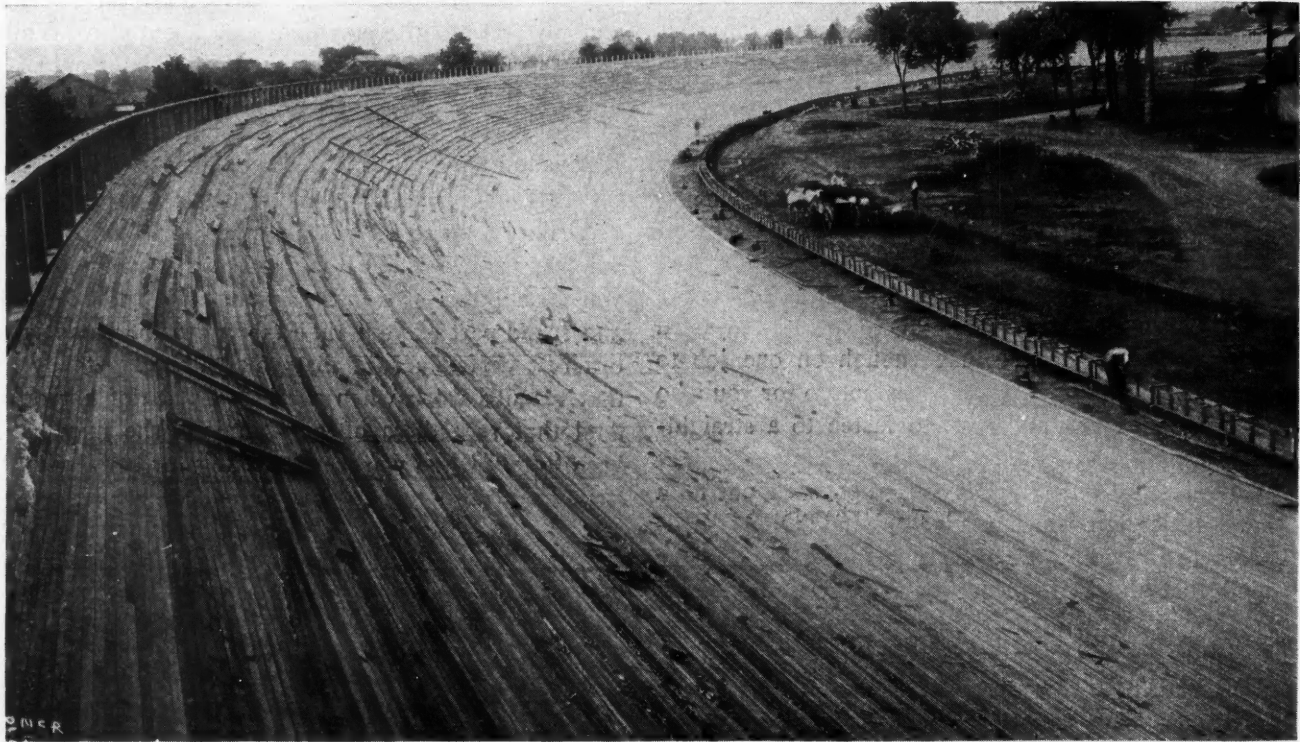
One Huge Turn on the New Sheephead Bay Speedway. The Banking Arises to a Height of 26 Feet. The Outer Rail of the Steel Framework Shown Will be Filled with Concrete to Form a Retaining Wall.
