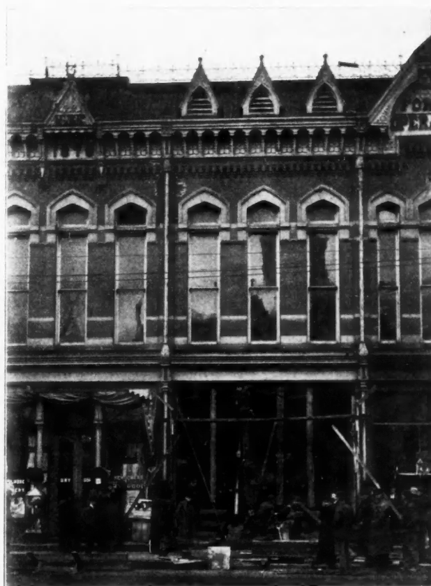
Fig. 3. This Shows Shoring Store Front so that New Entrance and Front Can be Put in. The Jack Posts are Placed so that Clearance is Given for the New Columns.
