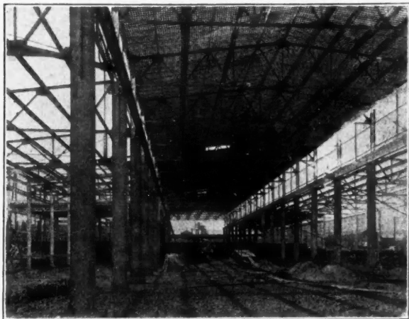
The Taylor-Boggis Foundry Co., Cleveland, Ohio. Contractors, John Gell & Son, Architects, Cleveland Engr. Co.
