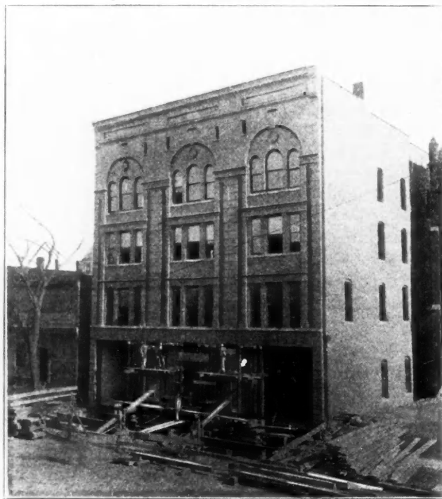
Fig. 1. Shoring Building. Notice Front Has Been Raised 8 Inches Higher Than the Piers.
