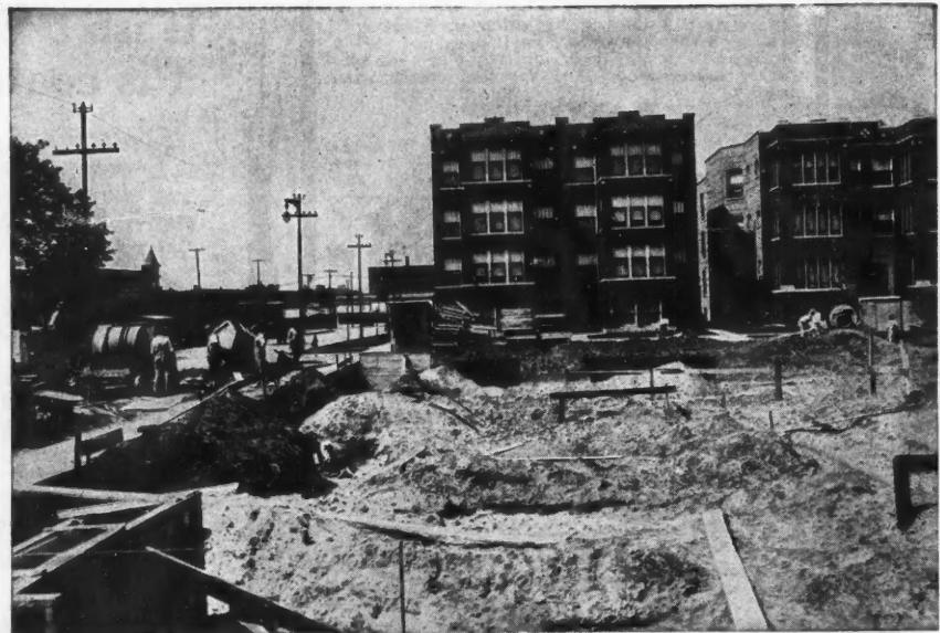
Bundo Bros., Chicago, Contractors, Using "The Standard" Low Charging Mixer on Apartment Building Foundation.
