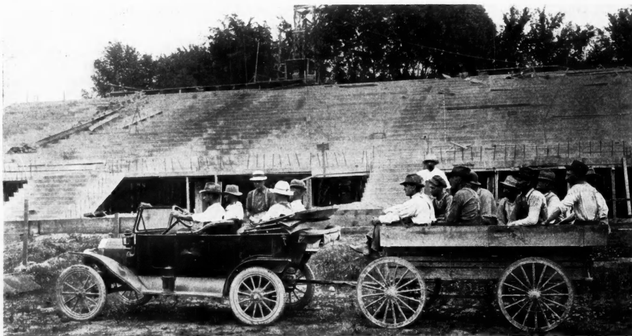
Hanneman Bros., Detroit, Mich., Contractors, Hitched a Miami Trailer to their Ford Car and Hauled a Crew of 15 Men, Night and Morning, to this Grandstand Job 20 Miles Distant.
