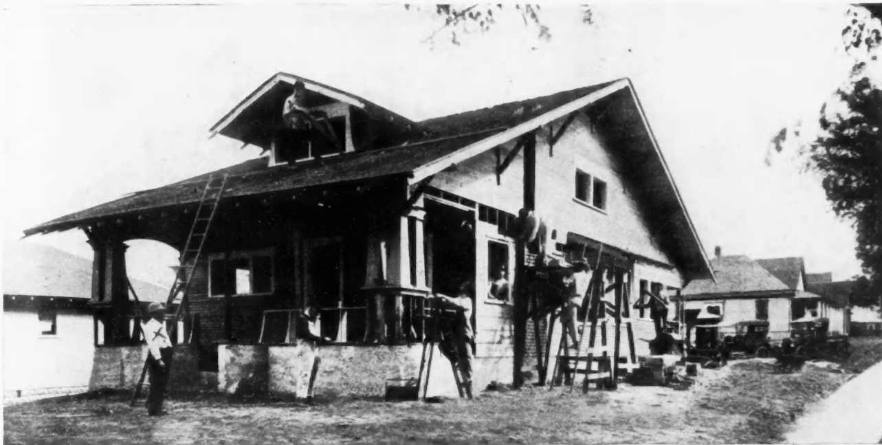
A Typical Bungalow Building Scene from Contractor Brown (by the Ladder) and His Power Equipment (in Background at Right).
