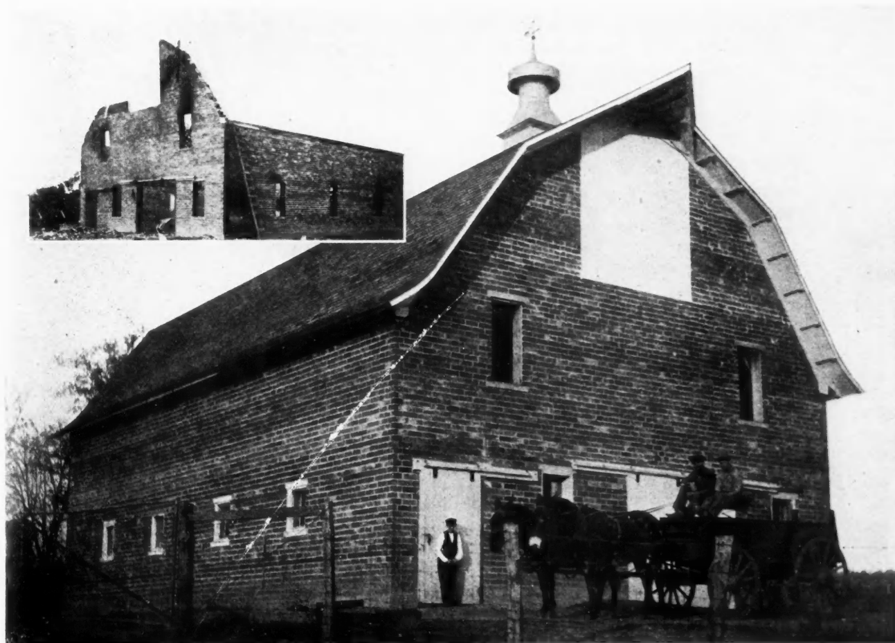
This Barn of clay block construction, located near Van Meter, Iowa, was filled with seventy tons of hay, which burned the interior and destroying the roof. The tile walls were very little damaged, and the "remains," as illustrated in photo inset, were restored to original usefulness at a fraction of the original cost of the building. An interesting side light to this circumstance is the fact that the owner collected full insurance as for a complete loss before starting to rebuild.
