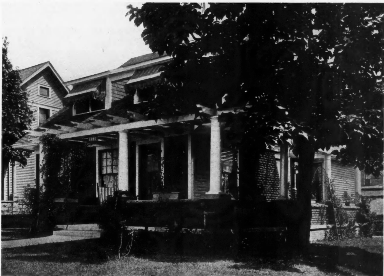
The Transformation Brought About by the Construction of a Pergol Porch with Face Brick Base and Wire Glass Roof is Clearly Evident in This View.
