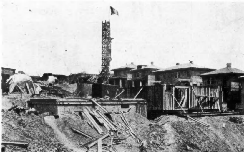
One Hundred Dwellings of Poured Concrete Construction Were Put Up as a Unit at Donora.
