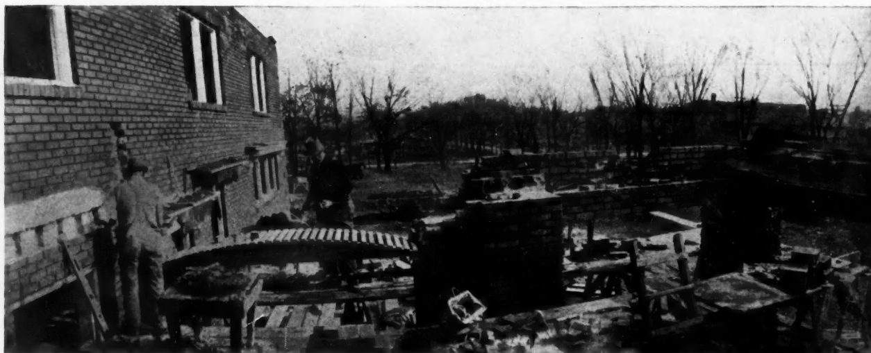
Brick Masons Lay Up Their Walls Carefully and Fashion Strong Arches Over Temporary False Work or Centers.
