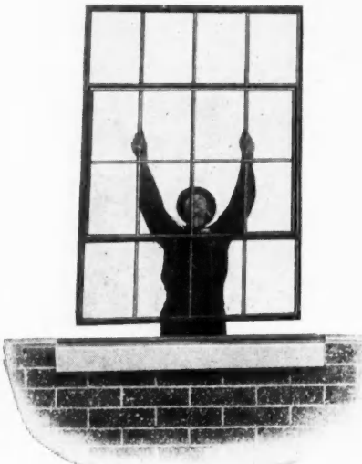
One Man Can Lift a Steel Sash Unit and Set it in Place on the Sill.
