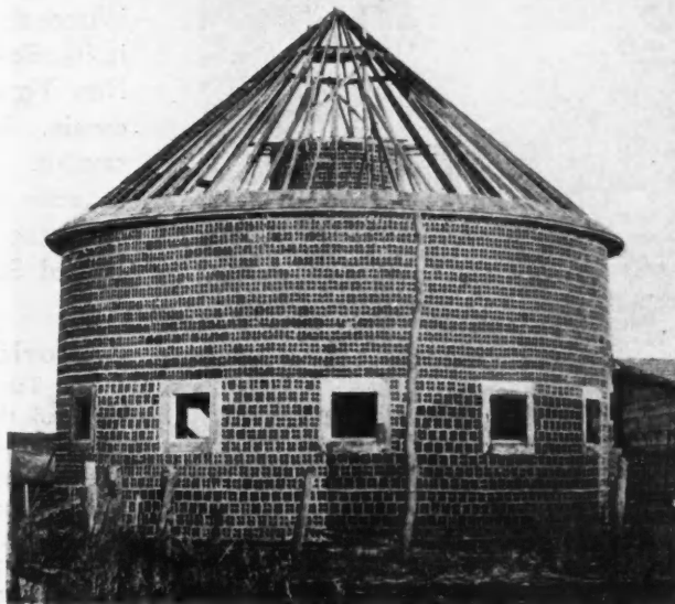
11,000 Bushel Ventilated Tile Corn Crib Being Built on Farm of N. B. Kinnick, Near Adel, Iowa. This is an Example of Safe Housing for the Precious Corn Crop.
