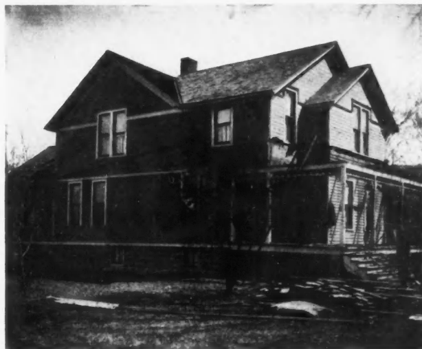
The Contractor Is Just Beginning the Remodeling Process by Tearing Off the Old Porch.
