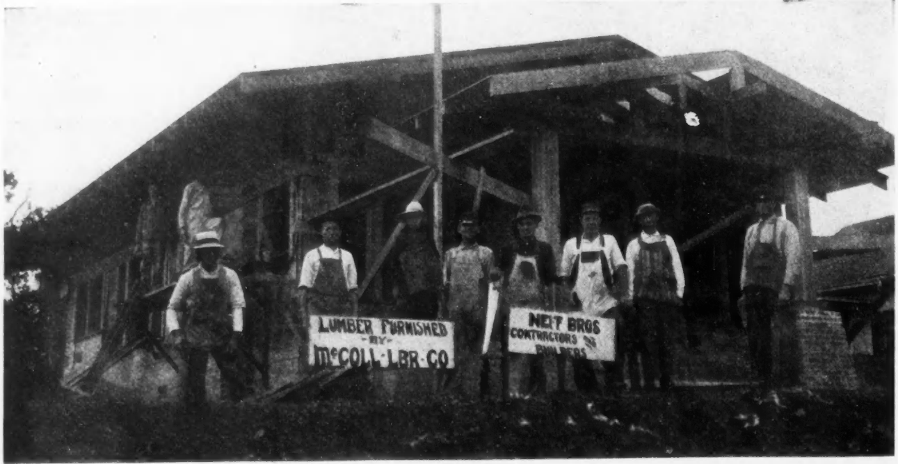
Neff Bros. and Gang on a Good Looking Bungalow Job at Redfield, Iowa.
