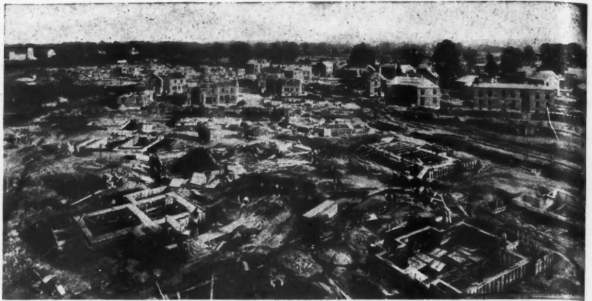
General View of the U. S. Shipping Board Building Project at West Collingswood, N. J.
