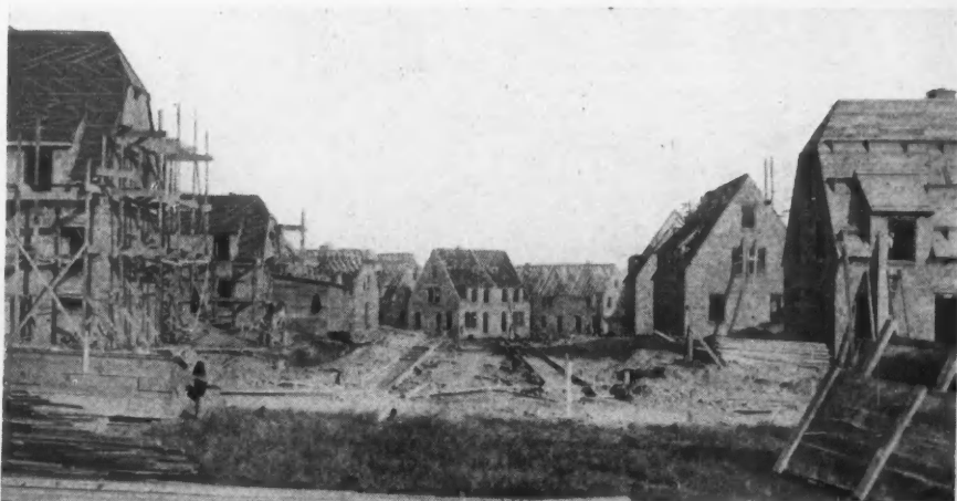
Hollow Tile Houses for the United States Shipping Board at Dundalk, Md., for Workers in the Bethlehem Steel Co. Plant.
