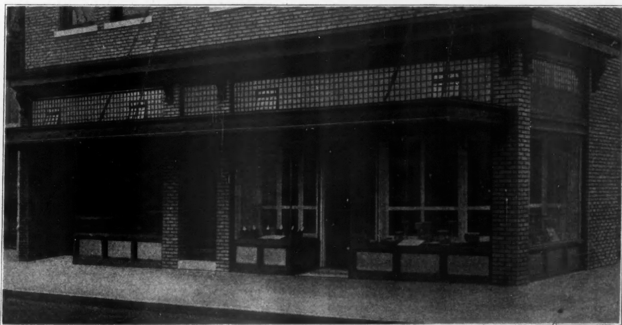
Here is the Same Brick Building After the Contractor Put in a New Front. It Will Be Noticed That a Window Was Added at the Side and That Brick Columns Set Off the Windows and Give the Structure a More Substantial Look.
