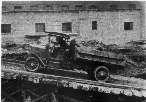
Removing the Dirt from a Building Excavation Is Another Use for Motor Trucks in the Building Industry. This 5-Ton "G. M. C." Is Hauling Seven Tons Up a 16 Per Cent Grade.
