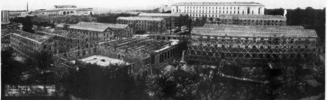
General View of the Dormitories for Government Clerks at Washington, D. C. This is one of the Government's construction projects in which hollow building tile was used.
