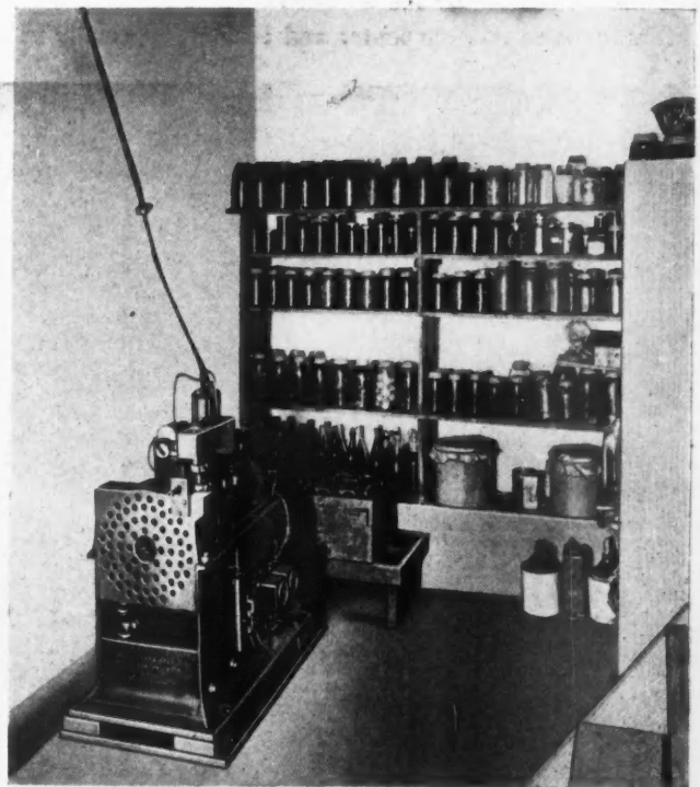
This Lighting Plant Was Installed Seven Years Ago in the Country Home of Henry Libben, Near Port Clinton, Ohio, and Has Given Him Excellent Satisfaction.
