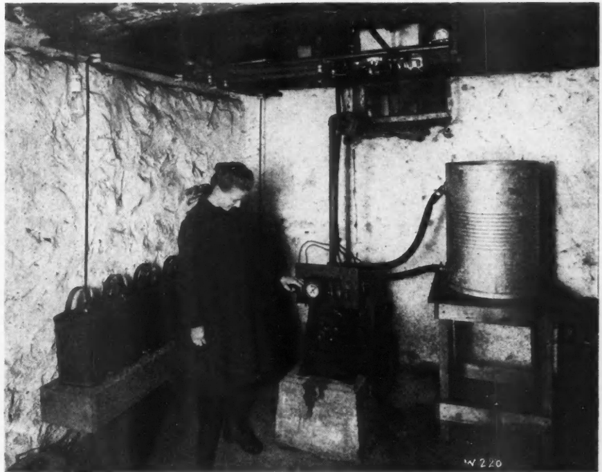
Some Idea of the Size of This Electric Lighting Plant Can Be Gained from This Picture. Placed in a Corner of the Basement, This Little Plant Supplies the Home and Other Buildings with the Greatest of Modern Conveniences.
