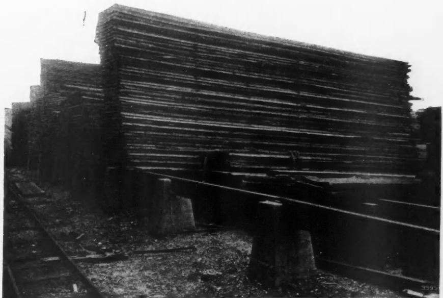
Foundations Are Strong and Properly Sloped, But Piles Are Too Close Together.
