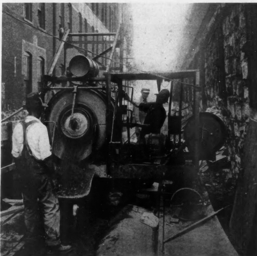
Laying a Concrete Retaining Wall in Advance of the Construction of a Large Building. This Portable Mixer Is Moved Along the Forms and Saves Wheeling.
