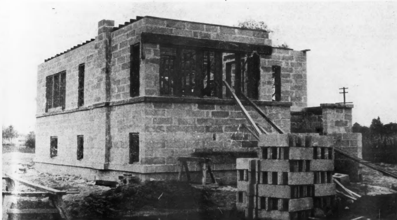
Figure 7. View of Partially Completed Concrete Block and Stucco Bungalow at Riverside, Ill. Forms for Monolithic Lintel and Sill Course are Still in Place. Block Walls of This Type Can Be Completed from Footing in About 2½ Working Days.
