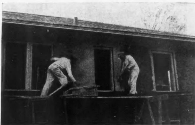
Figure 6. Applying the Stucco. Portland Cement Stucco, Properly Applied, Becomes Monolithic with the Body of the Wall. Recent Machine Methods of Applying Stucco Greatly Reduce the Cost Per Square Yard of Surface.
