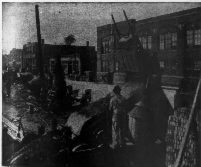
Combination Excavator and Loader at Work. Note Position Against Curb. The Trucks Do Not Have to Go Down Into Hole.
