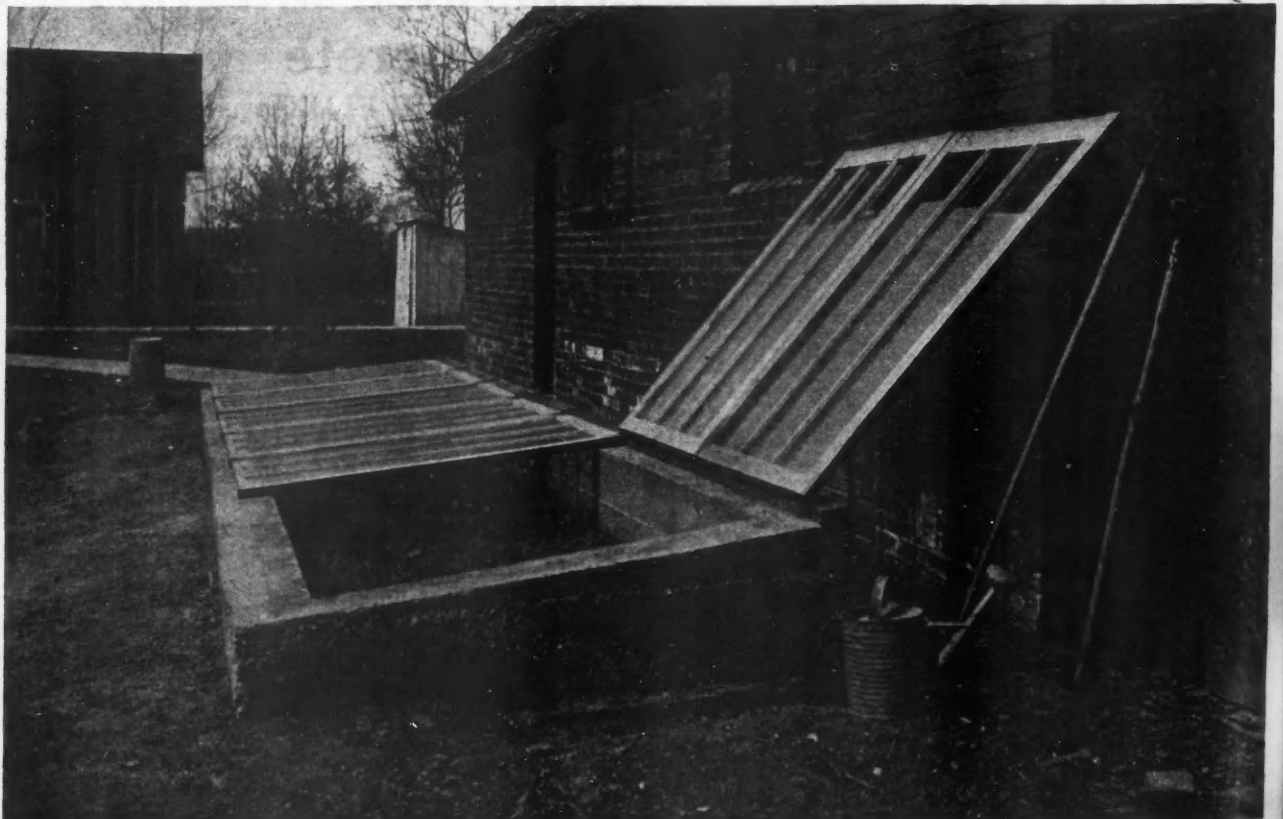
Newly Completed Concrete Hotbed in a Backyard Garden Patch of a Small City. An Enterprising Illinois Contractor Makes a Specialty of This Kind of Work and Has a Flourishing Business in the Spring Months. The Walls Are Six Inches Thick.
