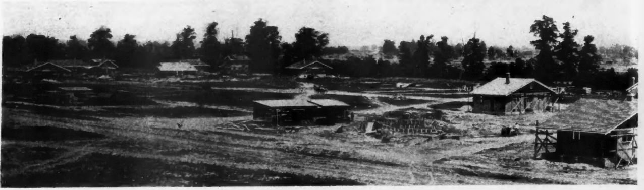
Mars Hill Housing Project Under Way. The Lafayette Motors Company Are Building 150 Homes for their Employees Near the Plant in Order to make them Contented and Reliable.
