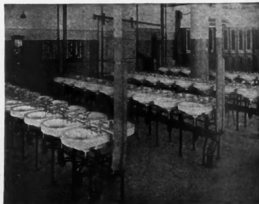
Modern Installation in an Up-to-Date Factory. Washrooms and Toilets Are Tremendously Important and Should Bear Close Study on the Part of Architects and Builders. Health and Cleanliness Make for Efficiency.
