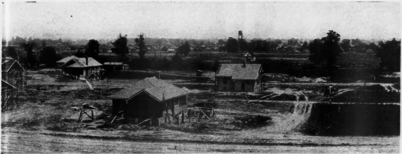
Concrete Tile Roofs Are the Feature of This Housing Project. These Roofs Are of Different Colors. The Homes Are Equipped with Electric Ranges, Light, Heating Plants and Modern Laundry. These Homes Will Be Sold at Actual Cost Plus Carrying Charges.
