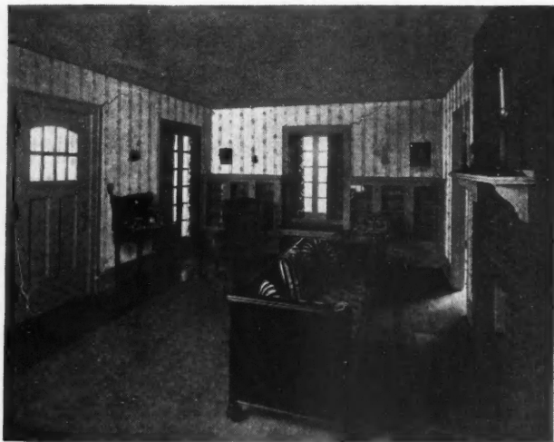
Photo of Room Before Using Wall-Board Which These Sketches and Material Lists Illustrate. Plans A, B, and C Show This Living Room Remodeled with Wallboard in Three Different Ways. Note the Wide Difference in Material Required and Cost.
