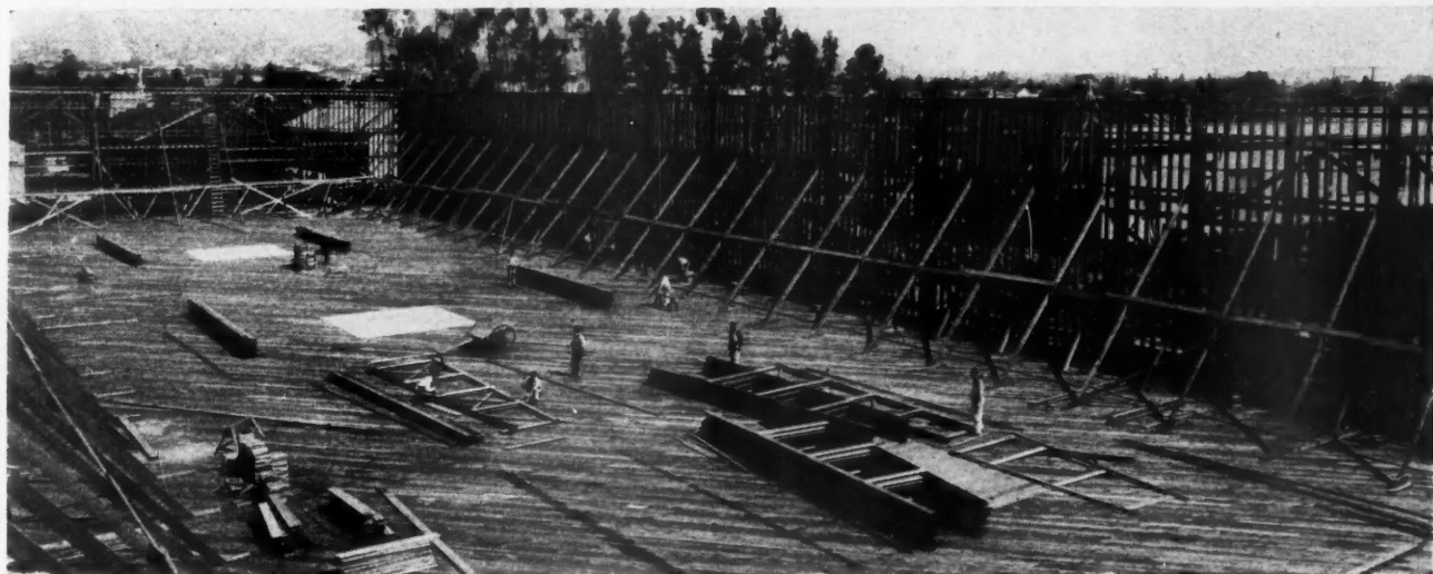
Largest Stage in the World, a Feat of Modern Building Skill. It Contains 36,000 Square Feet and Was Completed in Forty-Seven Days. It Is 300 by 120 Feet.
