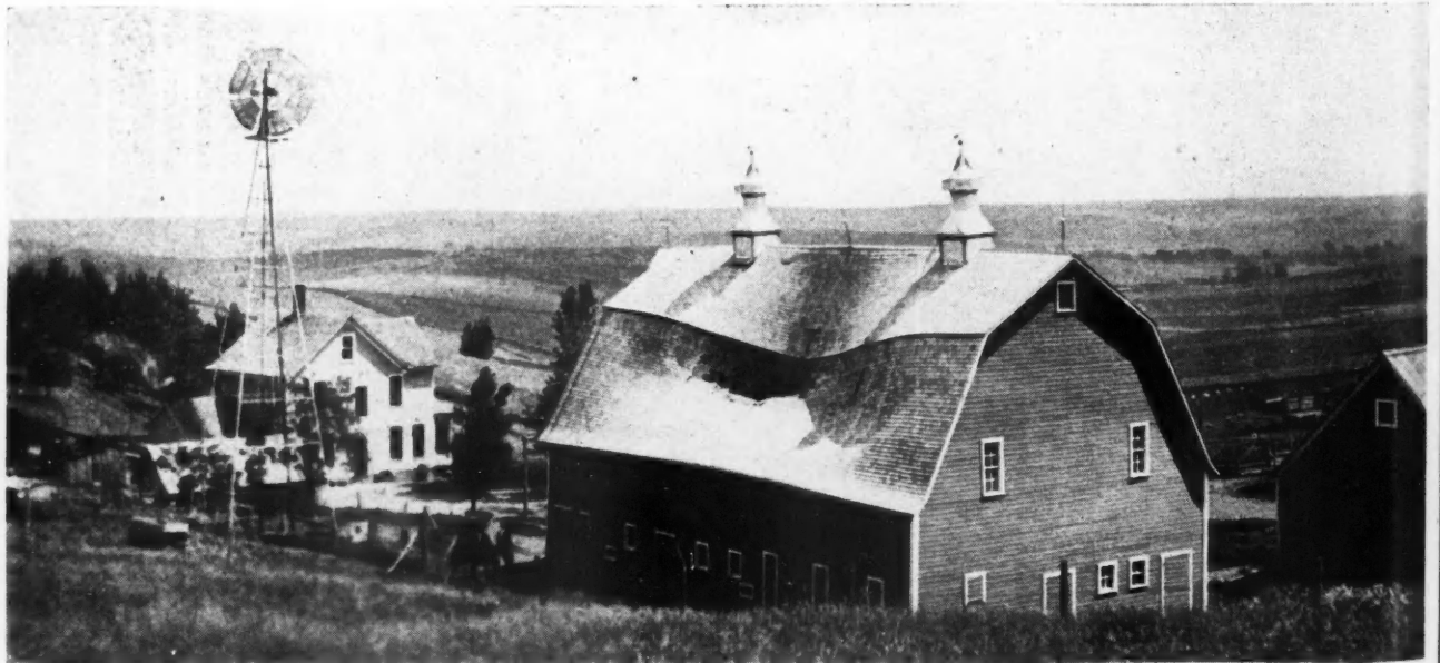
This Barn Was Unfortunate Enough to Get in the Way of a Tornado. The Weak Spot in the Roof Framing Collapsed Before the Terrific Pressure. Above is a Cross Section Drawing Showing Where the Break Occurred. This Type of Barn is Being Built Extensively Throught the West.
