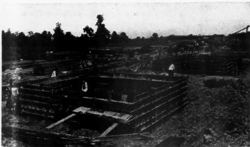
Steel Wall Forms Used on House Foundations in General Motors Co. Housing Project at Flint, Mich., Du Pont Engineering Co., Contractors. These Forms Are Taken Down in Units of Convenient Size to Transport to Next Foundation, in This Case 2 Feet Wide by 8, 10 or 12 Feet Long.
