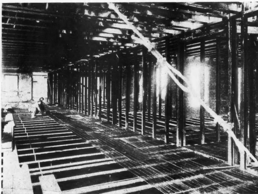
Steel Joist Floor and Steel Stud Partition Construction. The Workmen Are Placing Metal Lath for Firesafe Floor Slab.
