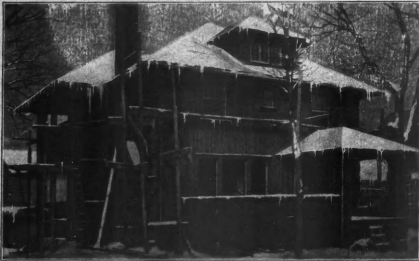
Residence—Wm. Mills, Cedar Rapids, Iowa. Architect—Wm. J. Brown. Stucco Contractor—Chas. R. Carpen er. Bishopric Base applied and left standing during Winter. Stucco applied in Spring.
