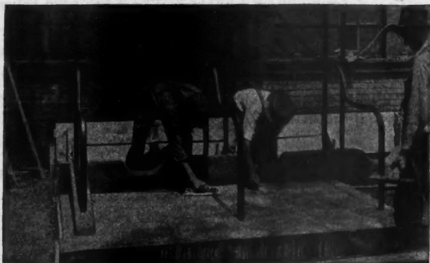
Fig. 5. Concrete for the Stall Platform Is Placed Next, Using a 1:2:3 Mixture, Finished With a Wood Float to Produce an Even, Non-Slippery Surface.
