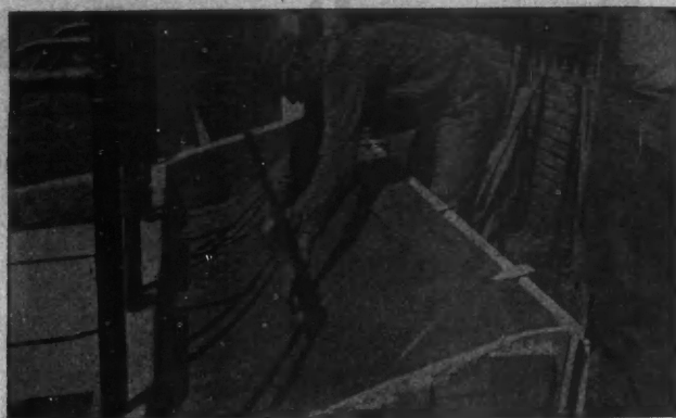
Fig. 7. Manger Templates Are Furnished by Manufacturers of Barn Equipment, and Should Be Removed Before the Concrete Has Hardened. Manger Is Finished With a Metal Trowel so as to Produce a Smooth Surface for the Cows to Eat From.
