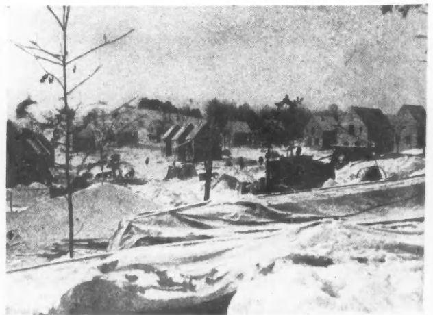
Fig. 3. A Number of Winter-Constructed Dwellings, With the Concreting Apparatus in the Foreground. By Placing the Concrete Portions During Cold Weather Conditions, It Was Possible to Complete These Houses Before Spring, Furnishing an Immediate Outlet for Lumber, Glass, Plumbing Goods and Other Building Materials and Work for the Building Trades.
