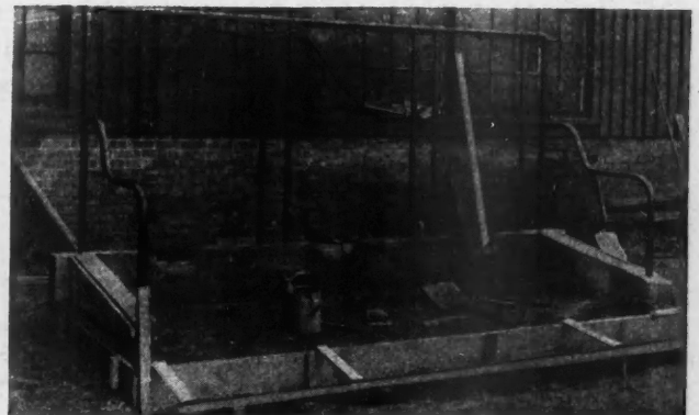
Fig. 4. Manger Curb Forms Are Removed and Concrete Placed for the Floor of the Litter Alley. The Gutter Between Litter Alley and Stall Platform Is Placed Later.
