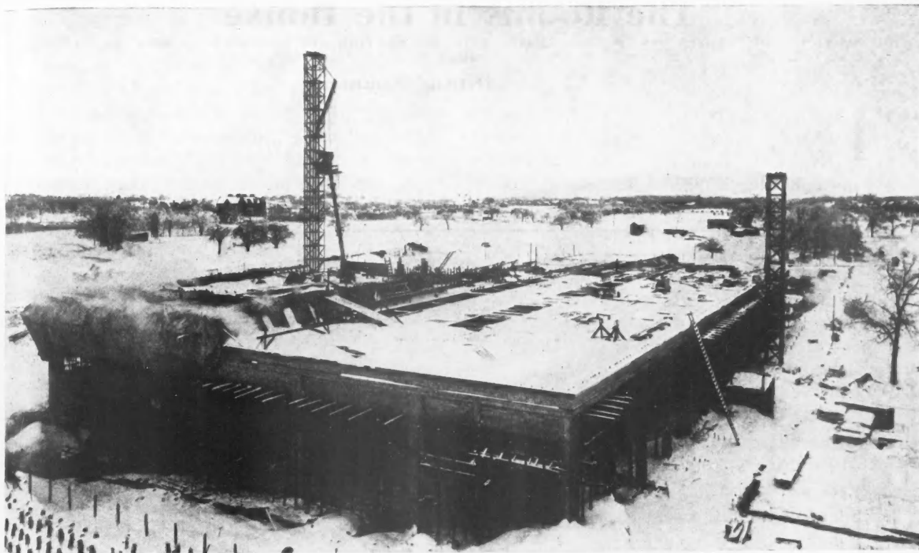
Fig. 4. The Newly Deposited Concrete in This Building Is Being Protected by Running Live Steam Under a Canvas which Encloses the Work. Steam Is Supplied by a Steam Boiler on the Job.
