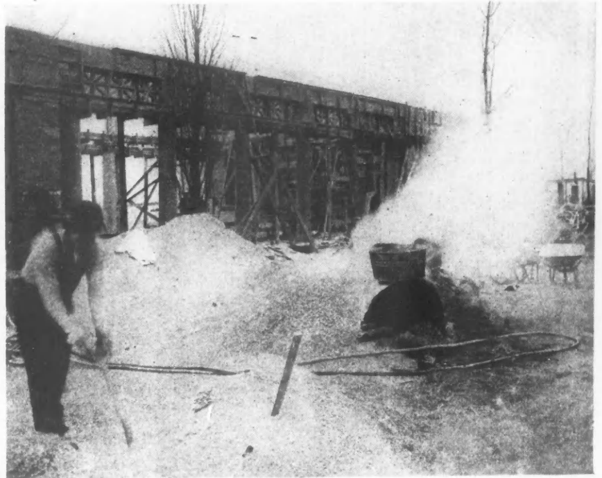
Fig. 1. Section of an Old Steam Boiler Employed for Heating Sand, Gravel and Mixing Water. This Arrangement Might Have Been Improved by Running a Coil of One Inch Pipe Thru the Improvised Fire Box, to Heat the Water.
