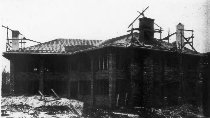
Fig. 3. An Apartment Building with Concrete Block Walls, Ready for Stucco Coats. These Block Afford a Rigid Base and Only a Minimum of Material Is Required for the Latter Operation, Since Wastage Is Small and the Coats May Be as Thin as Can Be Conveniently Applied.
