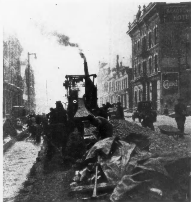
Big Paving Mixer Doing the Work of Many Men in Cold Weather. Mixers Have Become a Necessary Part of Builders' Equipment.
