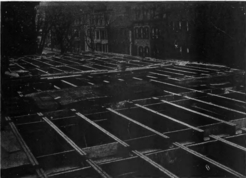
This Shows the Manner in Which Steel Joists for the Support of the Floor Slab Were Framed Into the Forms for the Reinforced Concrete T Beams. The resulting advantage is low dead-weight floor construction. The building shown is the Hagerstown, Md., Y. M. C. A.
