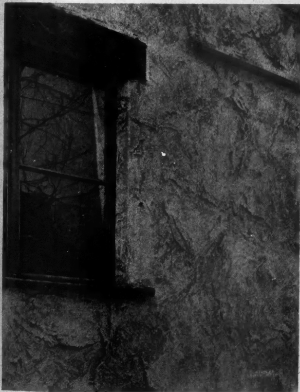
Close Up View of Characterful Stucco Finish; Also Note That Zinc, in the Form of Small Squares, Was Nailed to the End of Every Window Sill to Prevent Concentration of Water and "Tear Stains" or Streaks on the Stucco Below.
