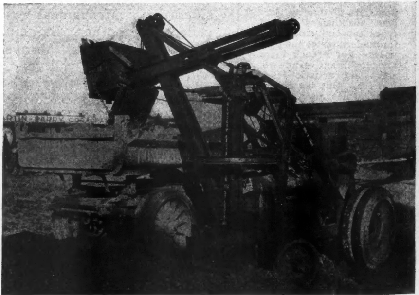
For the Builder Who Handles a Large Amount of Gravel, Crushed Stone or Other Material of a Like Nature, This Power Shovel Will Prove Useful. It also can be used for light excavating work.
