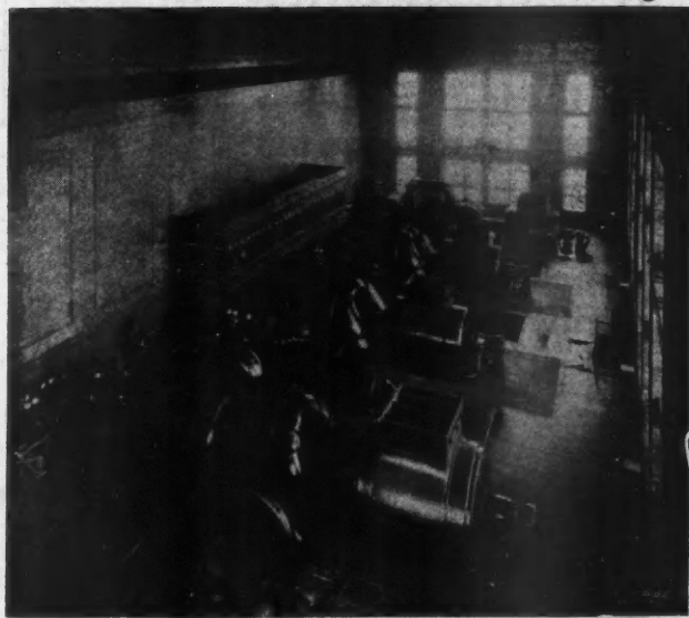
The Turbine Room in the New Hell Gate Central Station Which Supplies Electricity to a Part of New York City.
