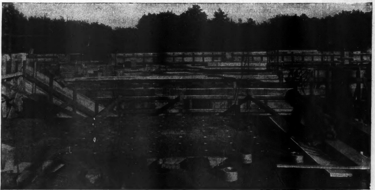
Rapid and Economical Building of Wooden Floors Over Concrete Is Possible Through the Use of Special Floor Clips Which Are Imbedded in the Concrete at the Time the Floor Slab Is Poured. Workmen place the clips by means of marked guide boards.
