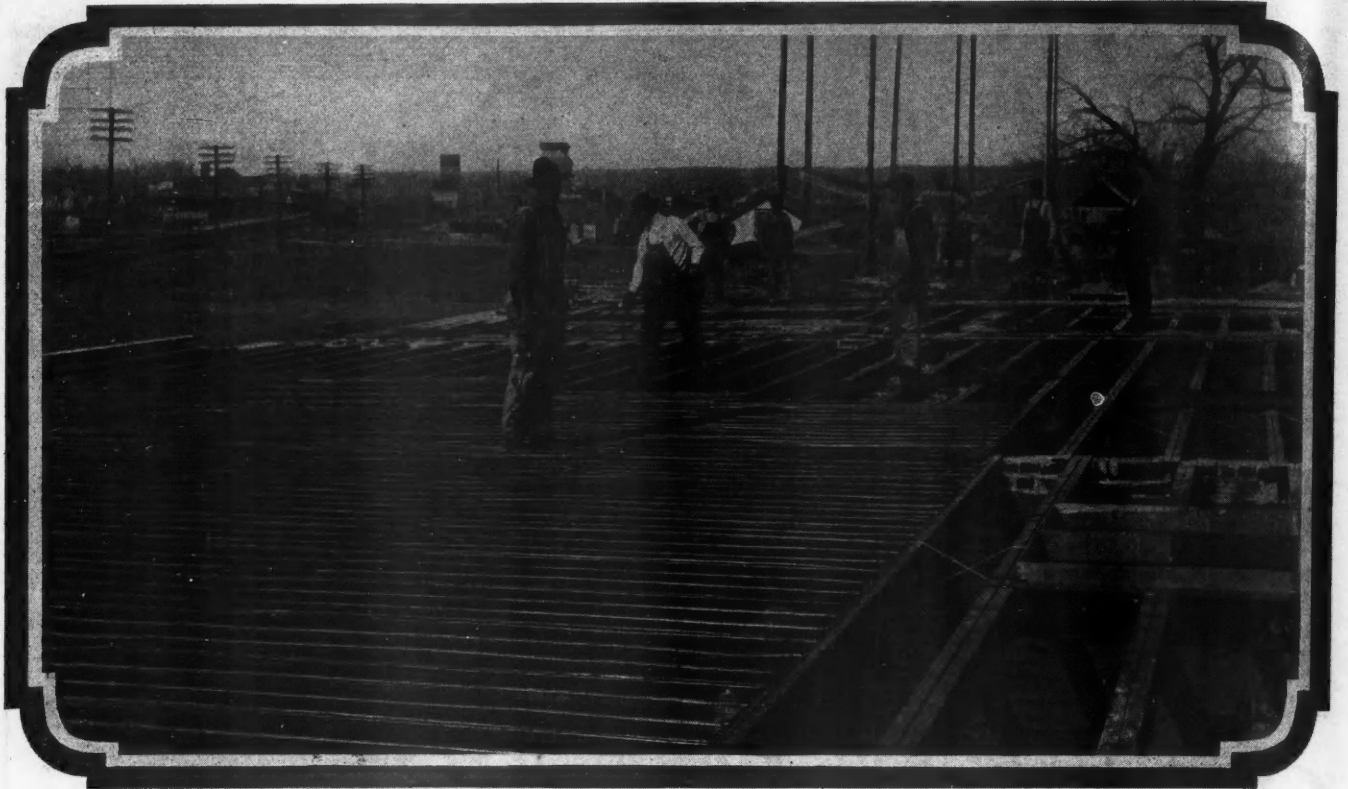
Applying the \frac{3}{8} " Ribplex to Metal Lumber joists. As the floor will be of concrete, wood nailing strips are not needed.
