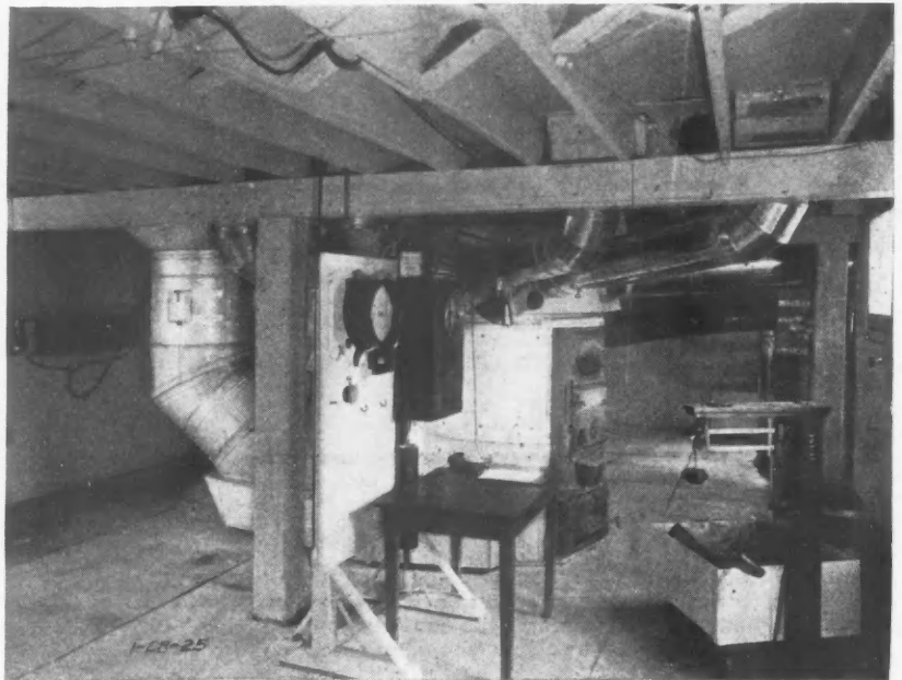
Furnace Installation and Part of the Testing Equipment Installed in the Warm Air Heating Residence. The equipment is complete from a scale for weighing the coal used up to the most elaborate instruments.
