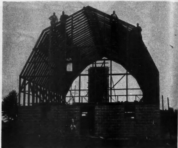
The Owner Has a Right to Be Proud of This Barn, for Even at the Stage of Construction Shown Here It Is Plain That It Is a Truly Modern Building.
