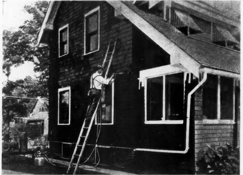
Exteriors of Small Houses May Be Painted With the Spray Gun in a Fraction of the Time Required for Brush Work.
