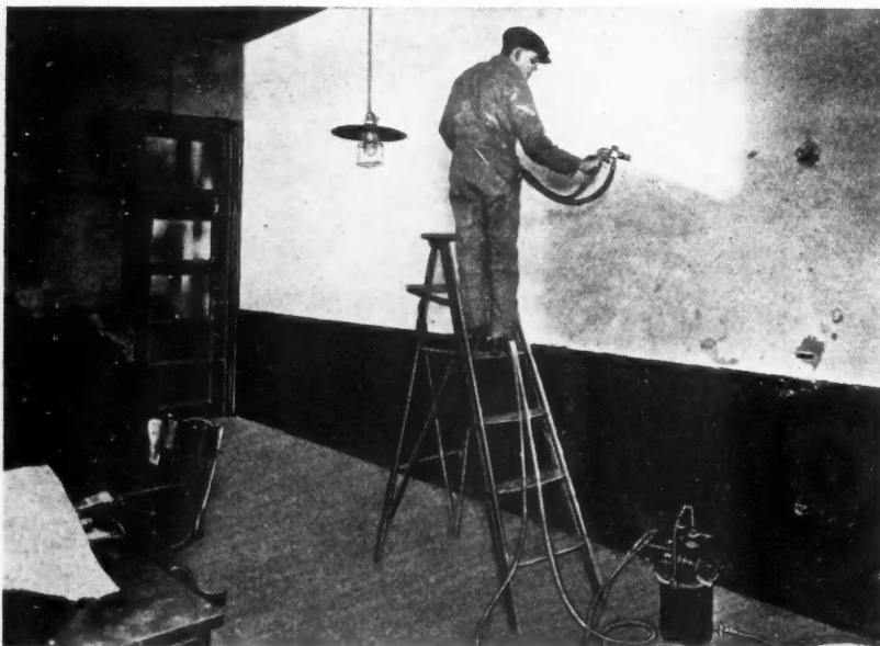
The Speed With Which Office and School Interiors Can Be Painted With Mechanical Equipment Reduces the Length of Time Necessary to Complete the Job.
