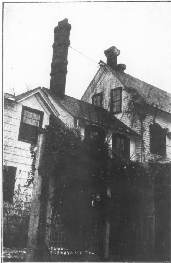
Fig. 3. A 50-Foot, Oblong Chimney, the Flue Area of Which Was Too Small to Afford a Good Draft. Three additions were made to obtain sufficient height to create a satisfactory pull.
