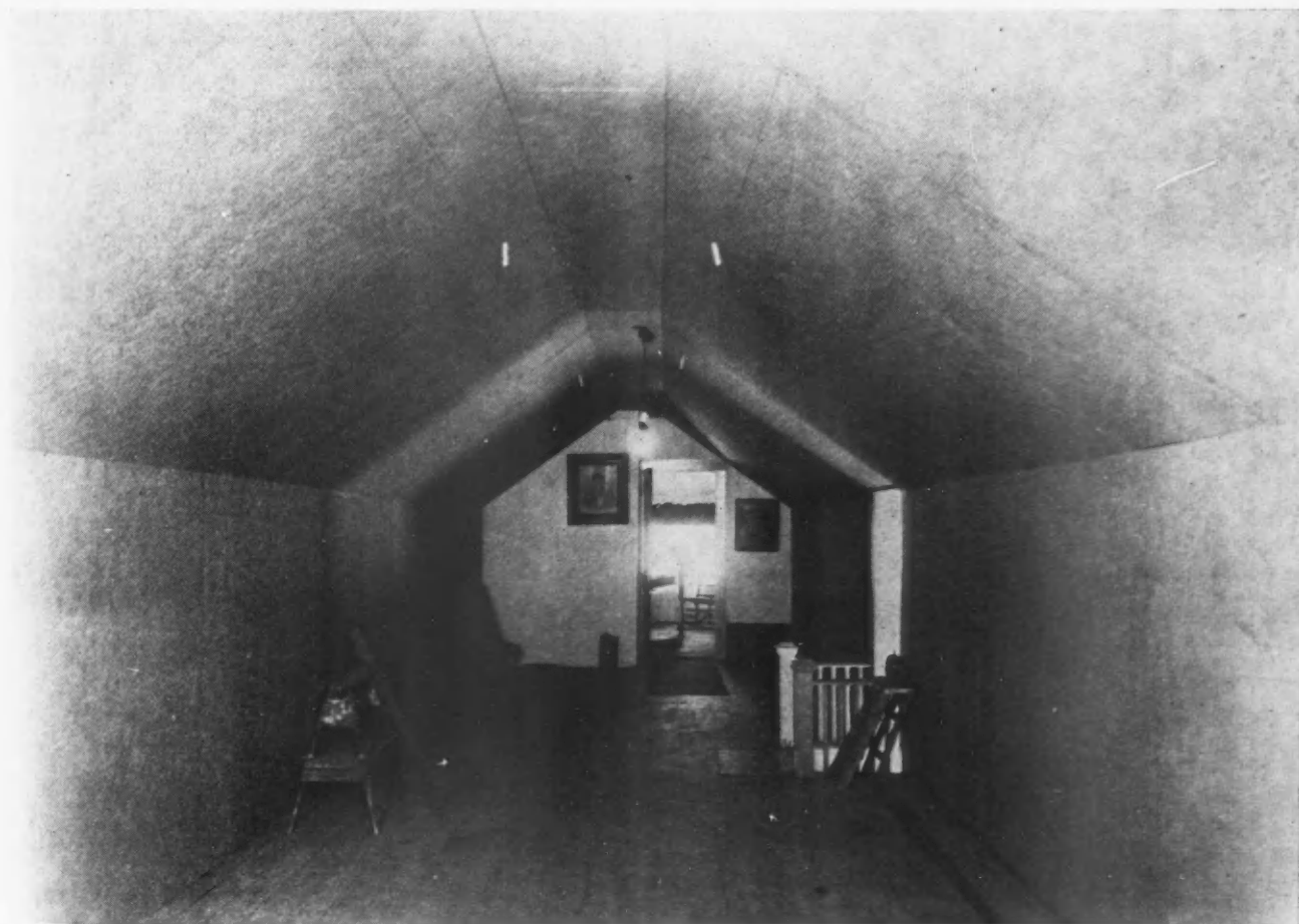
After Heating for One Season with a Gas-Fired Boiler, the Owners of This Chicago Bungalow Insulated the Attic with Cane Fibre Insulating Lumber as Shown in the Picture and Effected a Saving of 26 Per Cent in Their Gas Bills During the Following Winter.
