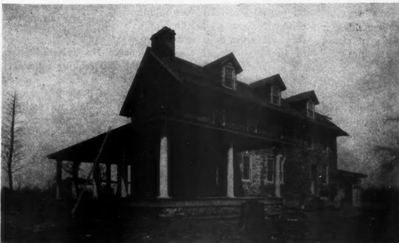
A Partly Finished Job of White Ribbon Pointing on an Old Stone Barn Built in 1775. It is still perfectly sound and since being renovated and remodeled has become one of the most attractive residences in Upper Darby, Pa.
