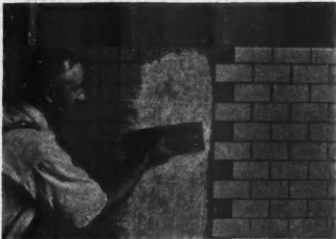
Laying Walls of a New Tile, Made of Vitreous, Porcelain Enamel Fused Onto Steel, Over an Insulating Base.
