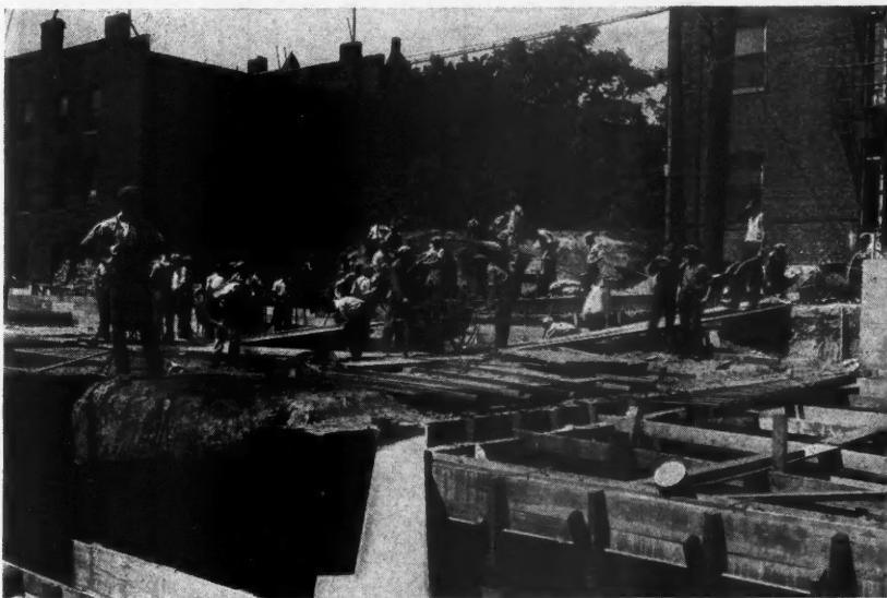
The Instructor in Each Trade Acts as Foreman Over the Boys Who Do the Actual Work and the Whole Job Is Supervised by an Experienced Contractor and Builder.
