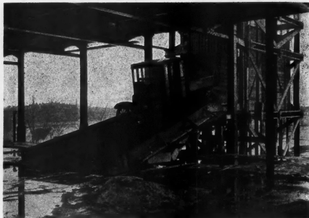
Truck Leaving the Elevator from Which It Carried the Materials to the Point Where They Were to Be Used.
