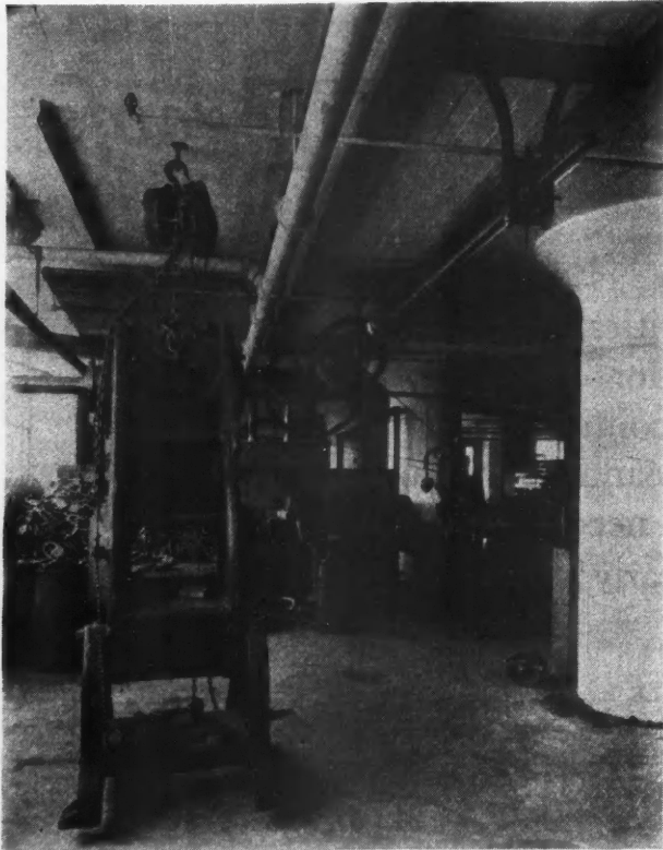
A Punch Press in the National Manufacturing Company's New Building Suspended from a Single Insert. The shafting and sprinkler system are also hung in the same manner.
