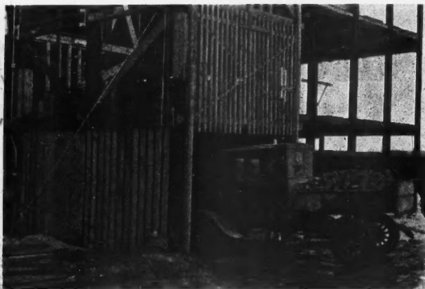
Truck Entering the Single Elevator Used for Raising the Materials for This Big Four-Story Building.
