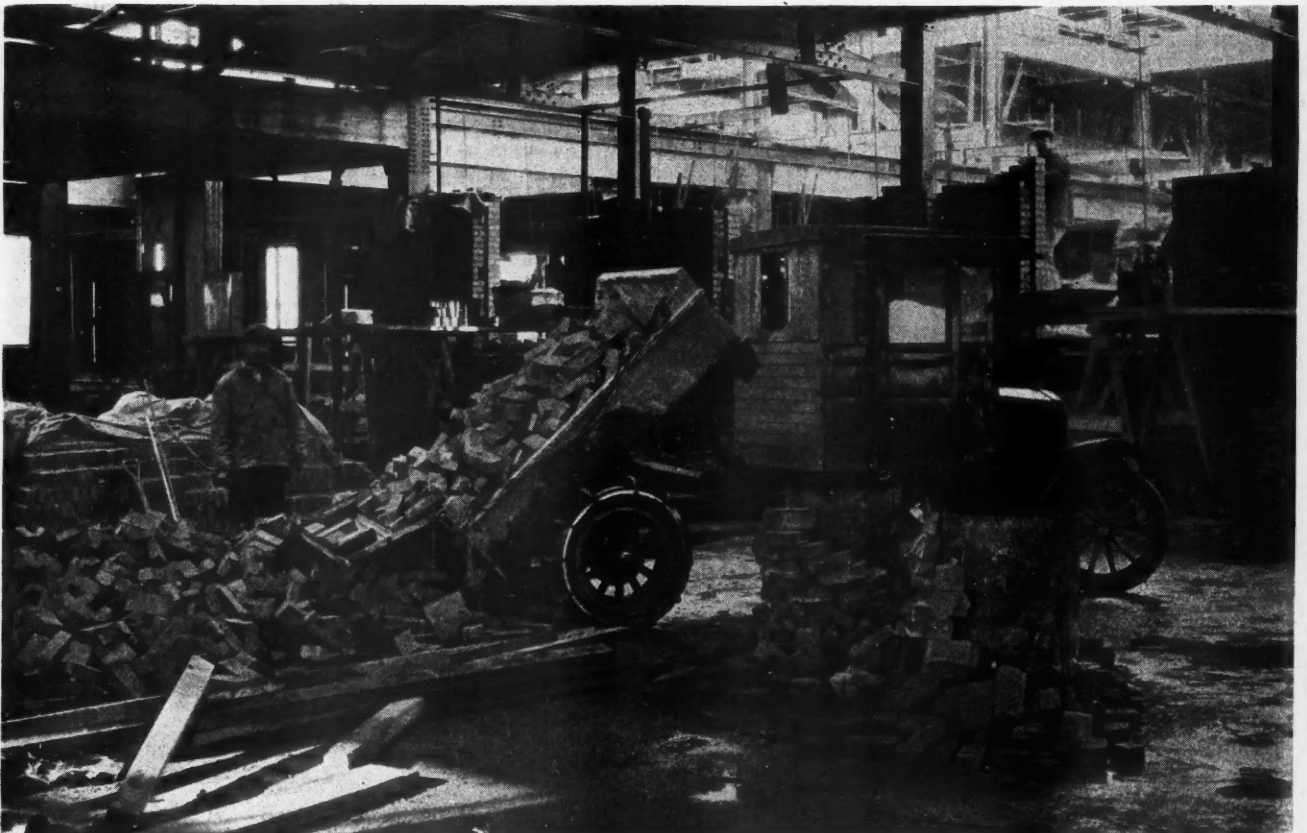
Delivering Brick by Motor Truck on One of the Upper Floors of the New General Office Buildings of the Massachusetts Mutual Life Insurance Company, a Highly Efficient Method of Handling Materials Which Was Introduced by the Turner Construction Company.
