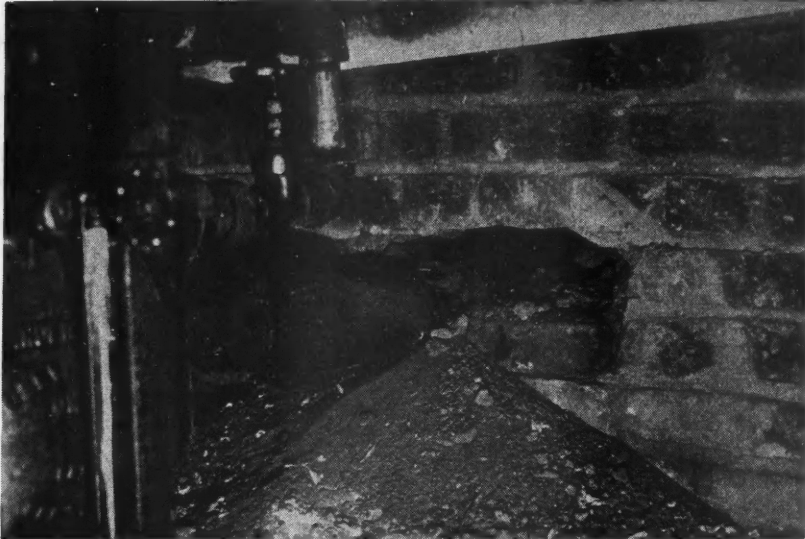
Unfinished Work Such as This Is Responsible for the Invasion of Rats in Many Modern Buildings Which Are Otherwise Rat-Proof.
