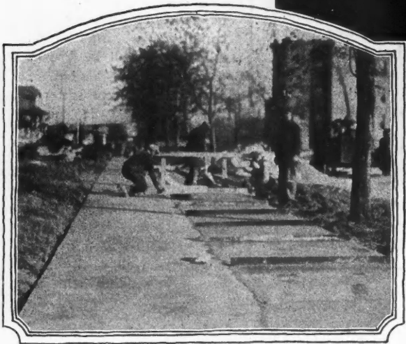
Sidewalk, Flossmoor, Ill. High-Early-Strength Universal concrete obtained by J. D. Smith, contractor, using standard Universal (not special) cement, the same quality Universal regularly handled and furnished by Darr Coal & Supply Co., Hazel Crest, Ill.
