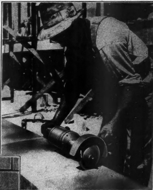
Cutting Random Ashlar strips to required length. Quick and easy because this electric carborundum saw is used instead of old mallet and chisel.
