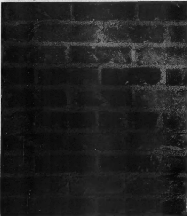
Running Bond, Flush Cut Joint, and a Wide Variety of Colors. Howell Gilbert, owner; Louise M. Gilleo, architect, Grand Rapids.
