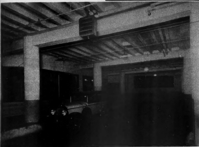
Entrance Driveway to the Baker Garage Showing Office Where Cars Are Checked In and Out, Also Doorway to "Foot Entrance." One of the unit heaters which heats the building shows in the immediate foreground.
