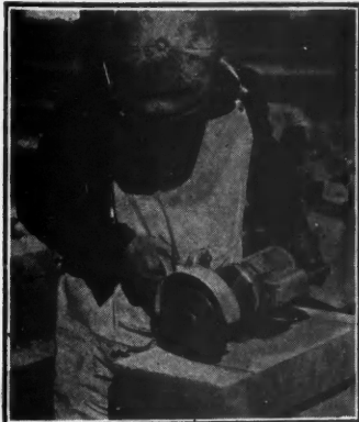
Portable electric saw replaces old mallet and chisel method of breaking stone. One man at ordinary wages now keeps six stone-masons busy!
