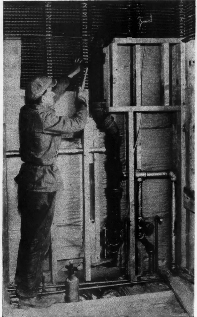
Quilt Insulation, the Proper Use of Brass Pipe and Metal Lath with Strong Framing Combined to Make the Concealed Portions of the Master Model Homes an "Honest Deal" on the Part of the Builder.
