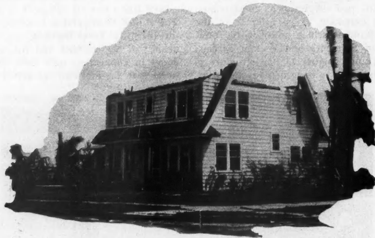
Lack of Anchorage of Roof to Side Walls Accounts for This Typical Roof Loss in the Recent Florida Storm. Good construction would have prevented this damage.
