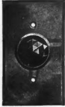
This Pilot Light Installed on a Stair Riser Warns if Basement, Garage or Other Lights Have Been Left Lighted.
