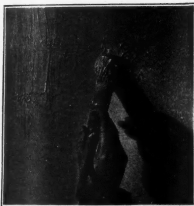
White Lead and Oil Plastic Paint Is Applied as Shown But with Flat Brush. Coating should be about equal in thickness to two ordinary paint coats.
