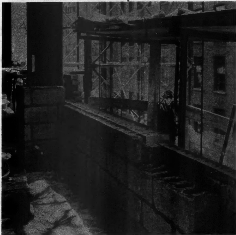
Exterior Wall of the 25-Story Integrity Trust Building Under Construction, Showing How Concrete Masonry Is Being Used for the First Time in Skyscraper Construction.
