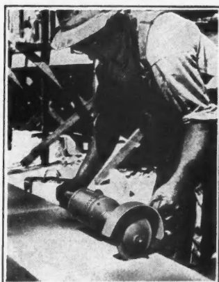
An electric carborundum saw, or an ordinary hand- or buck-saw, is used for breaking Indiana Limestone. One man keeps a number of stonemasons or bricklayers busy laying up stone.
