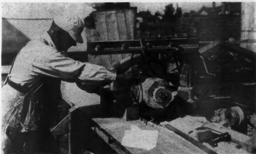
A Power Saw in Use on the Construction of a $200,000 High School in Calgary, Canada, by the Bennett & White Co., Ltd., One of the Contracting Companies Which Contributed Data Used in This Article.
