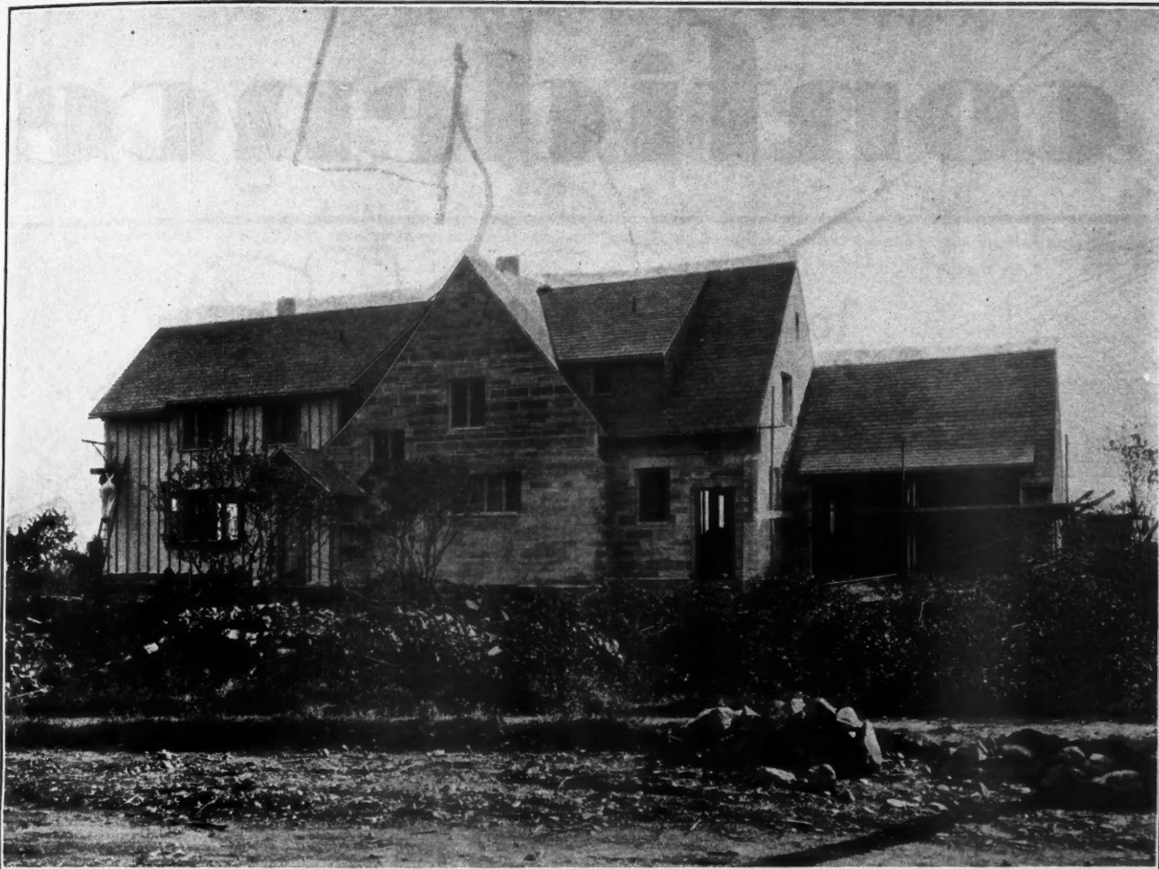
Residence, Marblehead, Mass., under construction. This house is being built of Old Gothic Indiana Limestone Random Ashlar with trim of Variegated Indiana Limestone. Wm. H. Quiner, Architect.
