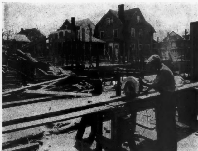
Here Dawson Bros., Ardmore, Pa., Contractors, Are Using a Power Saw to Turn Out 200,000 Feet of Lumber on an Apartment Job.
