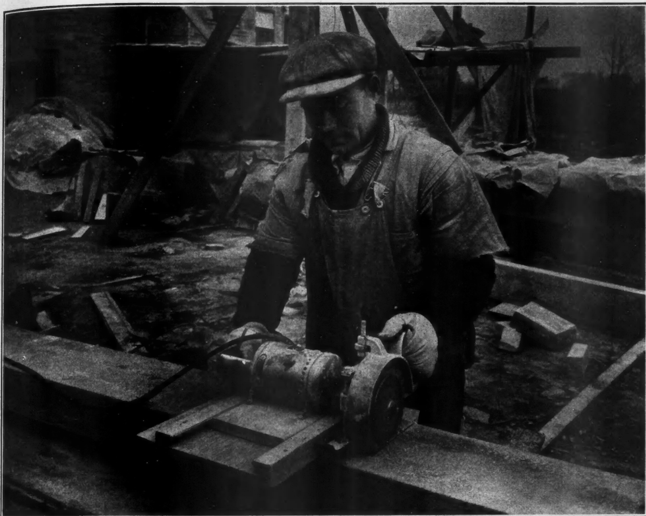
In breaking Indiana Limestone Random Ashlar, a shallow groove is made on one side of the stone strip by means of an electric portable saw or ordinary hand saw. The stone is then turned over and a tap with a mallet breaks it clean on a line with the groove.
