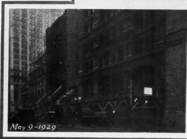
Below: On May 9th Wrecking Was Under Way. Tenants are still in the large office building.
