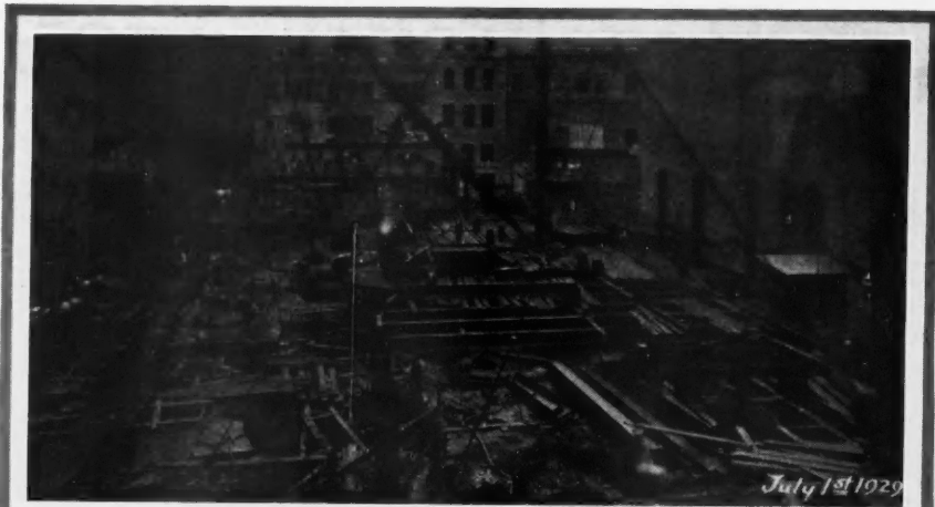
To Right: The Start of the Steel Erection July 1st, Demolition Debris Still Being Removed.
