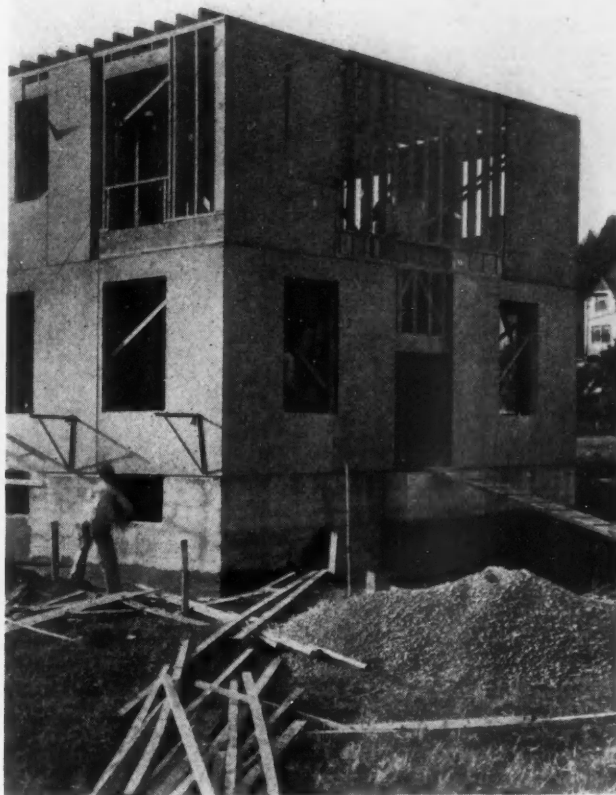
Sawing Out Window Openings in Large Panel Plywood Sheathing in Wuest House.
