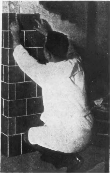
Applying the New Sheet Metal Tile by Pressing Against the Oil-Cement Coated Wall.
