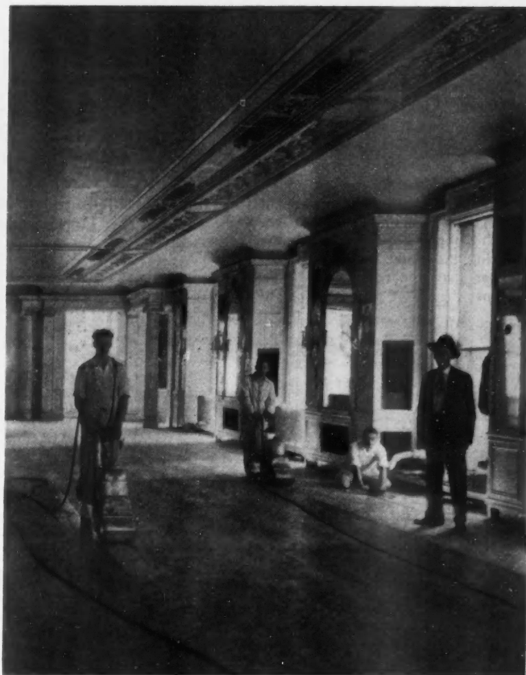
Instead of Working as a Cabinet Maker, as He Did For Many Years, Mr. Cunningham (Shown at the Right) Now Directs His Crew of Men in the Performance of Such Jobs as This One—Resurfacing the Floor of the Chrystal Ballroom, Book-Cadillac Hotel, Detroit.
