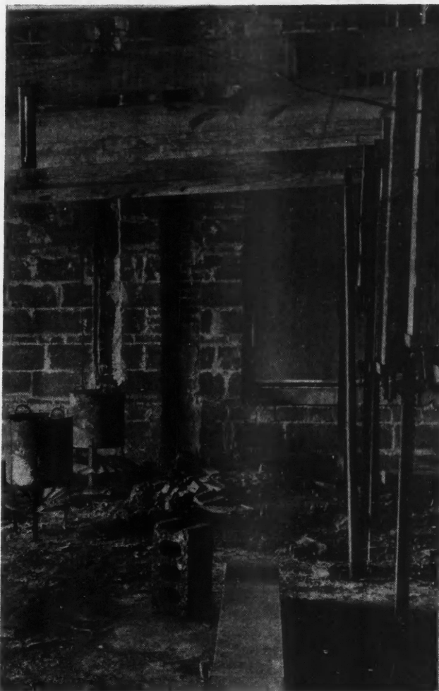
Heat supplied by salamanders and temperature checked by thermometer until concrete and mortar has fully set. Hinsdale Memorial building, Hinsdale, Ill.
