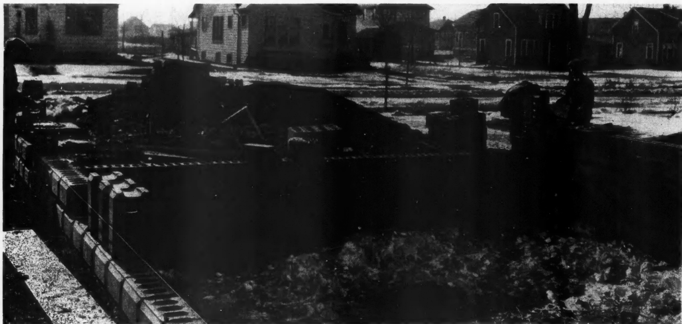
Laying up a concrete masonry wall for small home in Illinois, middle of January. Chas. Arbogart, builder.
