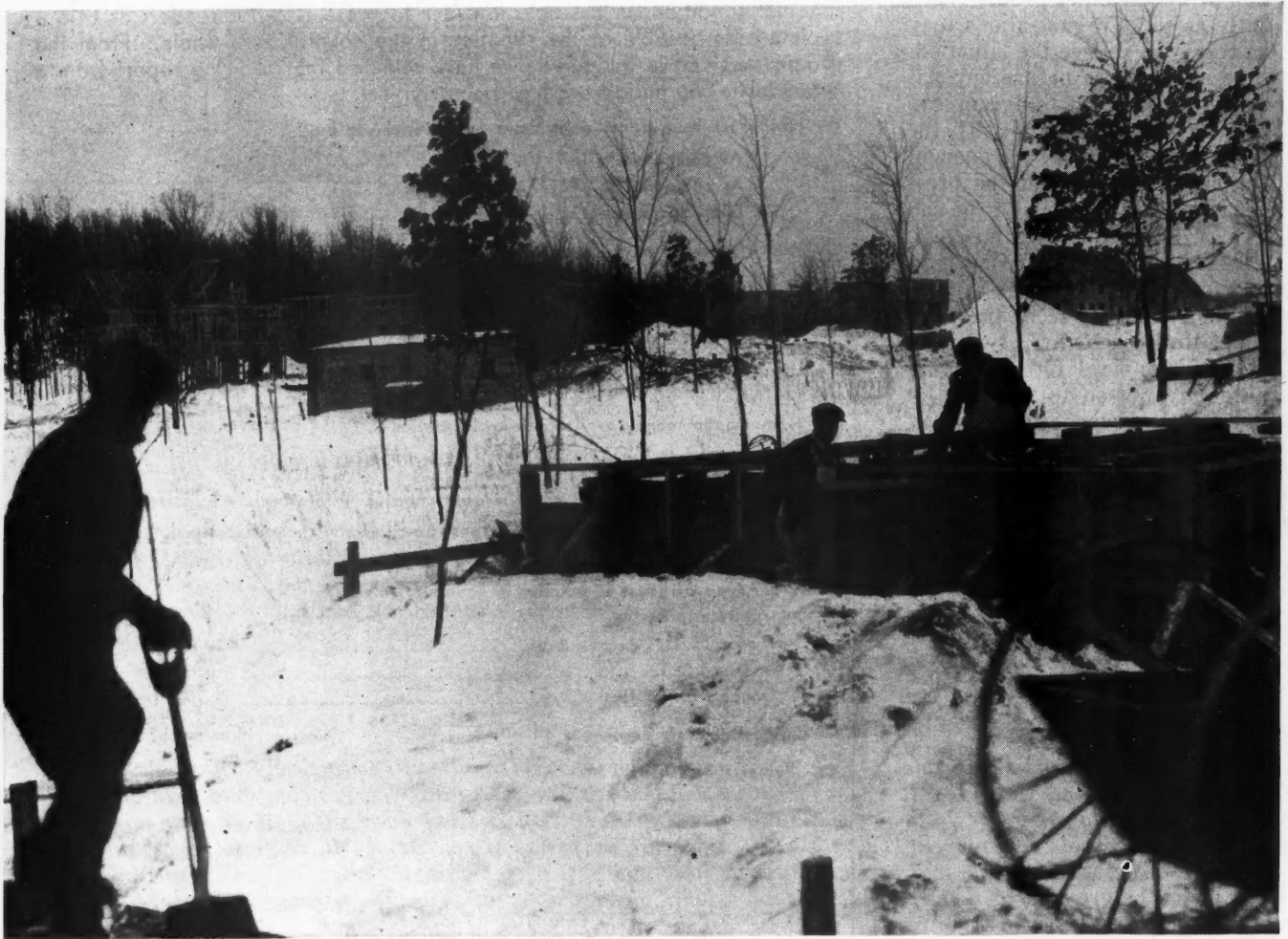
Home building done profitably in spite of snow on this Massachusetts project. F. T. Foley & Co., contractors.
