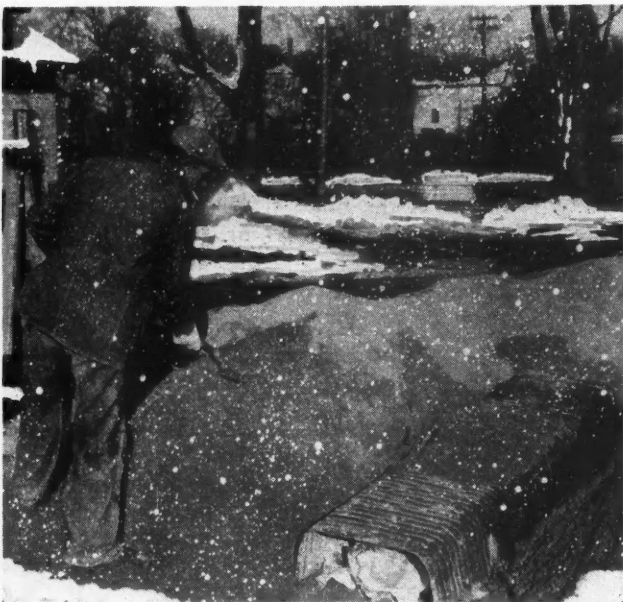
Preparing to heat sand for concrete by building fire under pan. Adams Const'n Co., Hinsdale, Ill.
