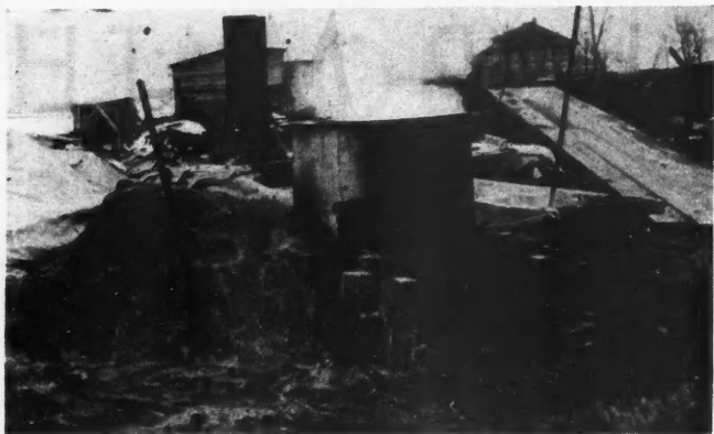
Heater made of concrete block and old tank to warm water and sand for concrete work.
