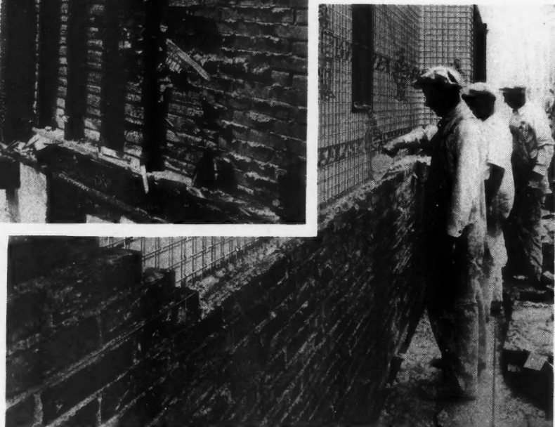
Below, Workmen Laying Brick for Reinforced Super-wall Slush the 1" Back Space Full of Mortar.
