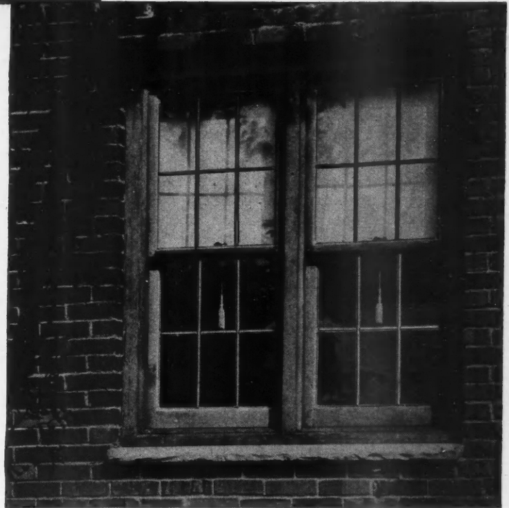
The exterior beauty of narrow mullions is apparent. The same narrow outside casings are used in all types of walls. More light or more wall space as desired. Narrow trim applied without expensive preparation of back of pulley box.
