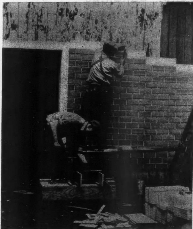
Applying the new brick siding made of asbestos and cement to an old structure
