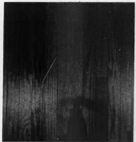
Figure 3—Crack resulting from use of a crooked board that was forced into place. Such pieces should not be used.
