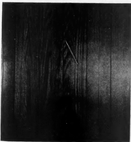
Figure 1—Results of moisture absorption when floor was newly laid. An even temperature of 70 degrees would have prevented cracks.
