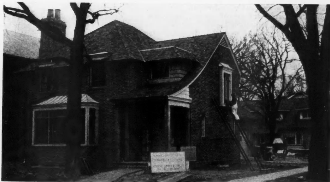
A "DRY INTERIOR" is the feature of this new home just being completed at Rockford, Ill., by Contractor J. H. Thomas. It was designed by Willis W. Hubbard, architect. Interior walls are of gypsum board with armored joints covered with canvas.
