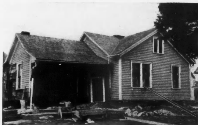
NEW FOUNDATION, A NEW FRONT PORCH and exterior refinishing are included in work going ahead on this house at Cascade, Ia. Considerable modernizing work is going ahead in Iowa and Illinois.
