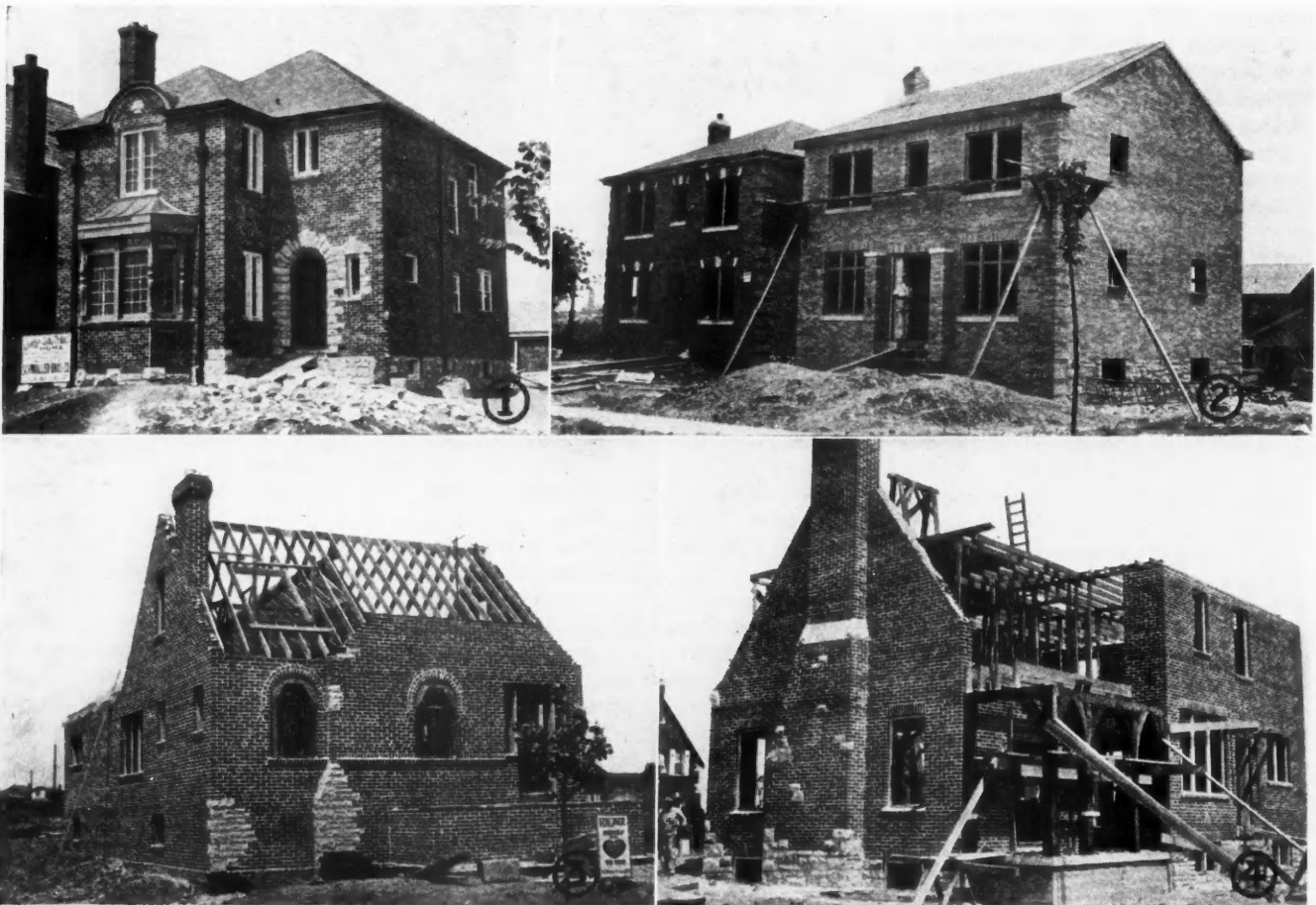
BUILDING ACTIVITY IN ST. LOUIS HILLS: 1—Schwaller Bros. are building this 6-room, insulated, gas heated home. 2—Two $9,000 houses being built for sale by contractor C. N. Williams. 3—A $6,000 house being built for sale by Harry Hardt. 4—Attractive English type brick home costing $17,000 being built for owner by contractor Arthur R. Darr. Increased activity by builders is expected.
